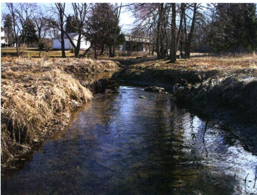
Figure 4-2. Typical conditions upstream of the south Market Street bridge showing moderately entrenched stream with minor bank erosion.
