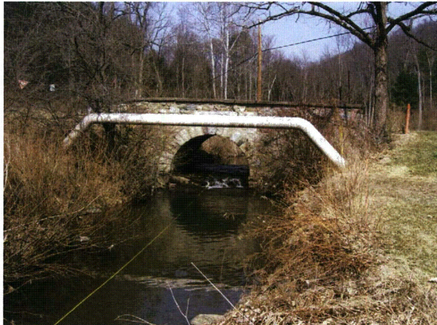
Figure 4-15. View of Beach Grove Road bridge crossing with elevated high-pressure gas line.
