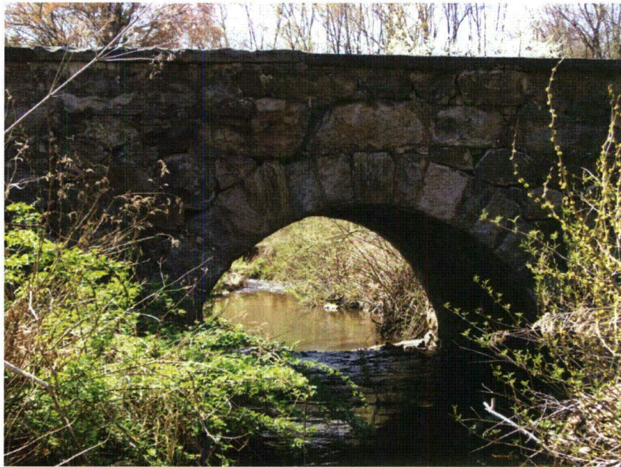
Figure 4-16. View of the Beach Grove Road bridge culvert (facing downstream). The undersized opening creates an upstream backwater condition during high flows, which limits sediment transport.
