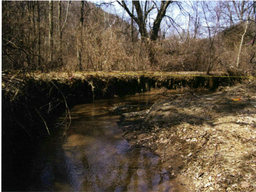
Figure 4-12. View of typical stream conditions showing bank erosion approximately 400 downstream of Beach Grove Road.
