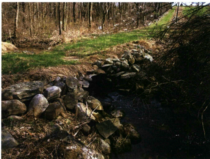
Figure 4-3. View of the culvert crossing along an existing farm access road, which provides the primary upstream base level control. This control structure prevents long-term vertical bed degradation upstream because of the fixed bed elevation of the culvert.
