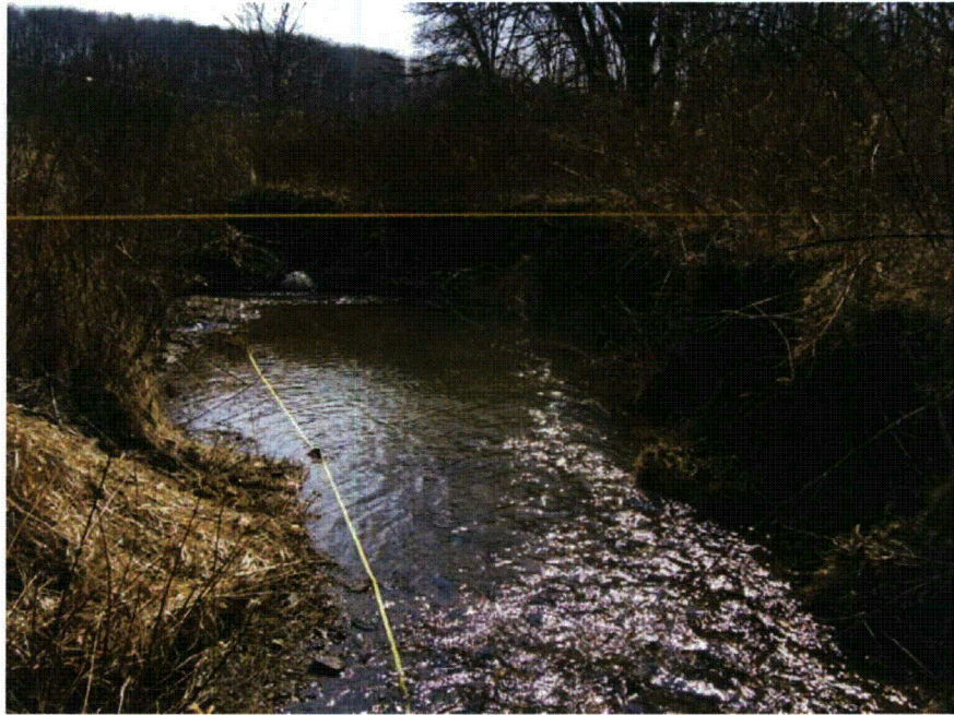
Figure 4-14. View of severely-eroded vertical bank immediately downstream of Beach Grove Road at a 90-degree bend to the left (facing downstream).
