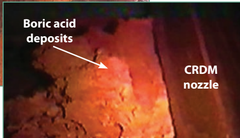
Figure 3b. Boric acid deposits accumulating near a CRDM nozzle (still photo of video taken during the 2000 refueling outage at DBNPS)
