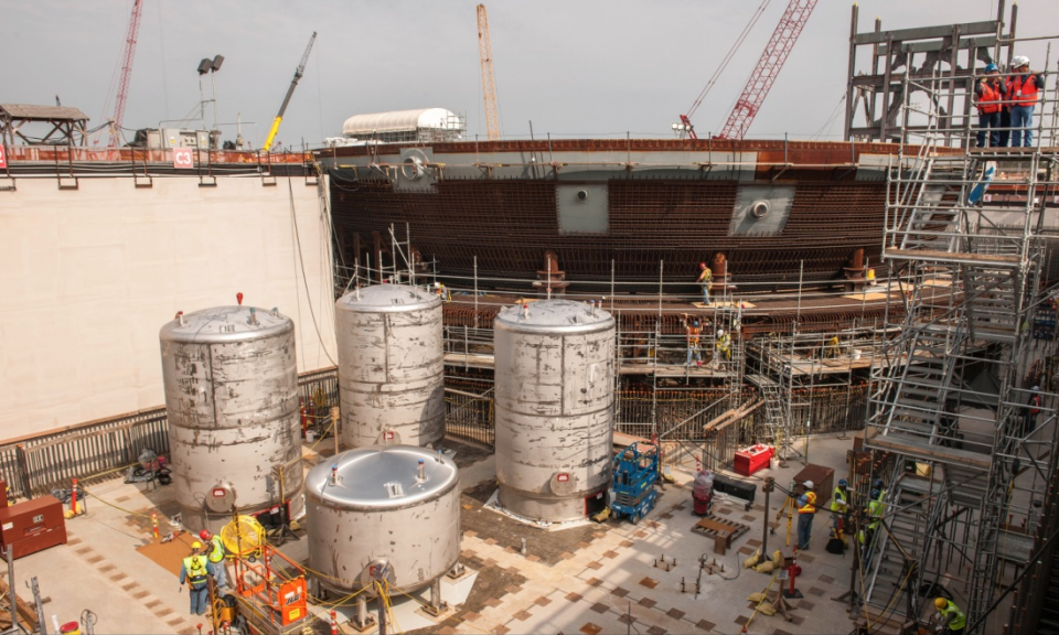
Plant Vogtle Unit 3 liquid processing tanks inside nuclear island
