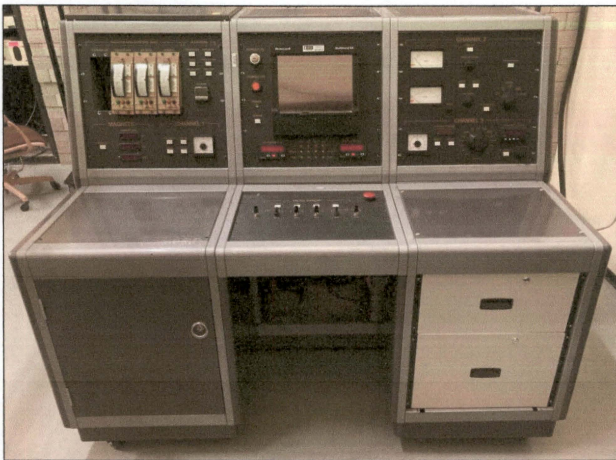
Fig. 4.2-1 AGN-201 Nuclear Reactor Control console
