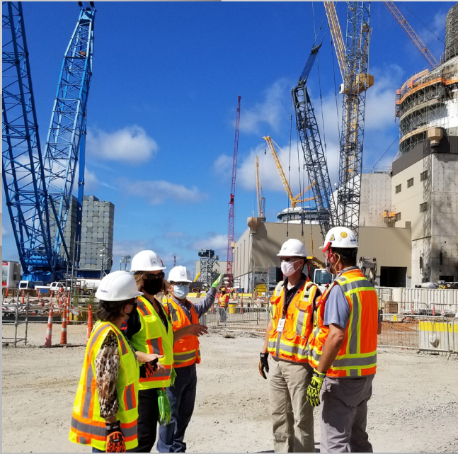
NRC inspectors keep a close eye on construction activities to ensure NRC regulations are being met at Vogtle Units 3 and 4 in Georgia.
