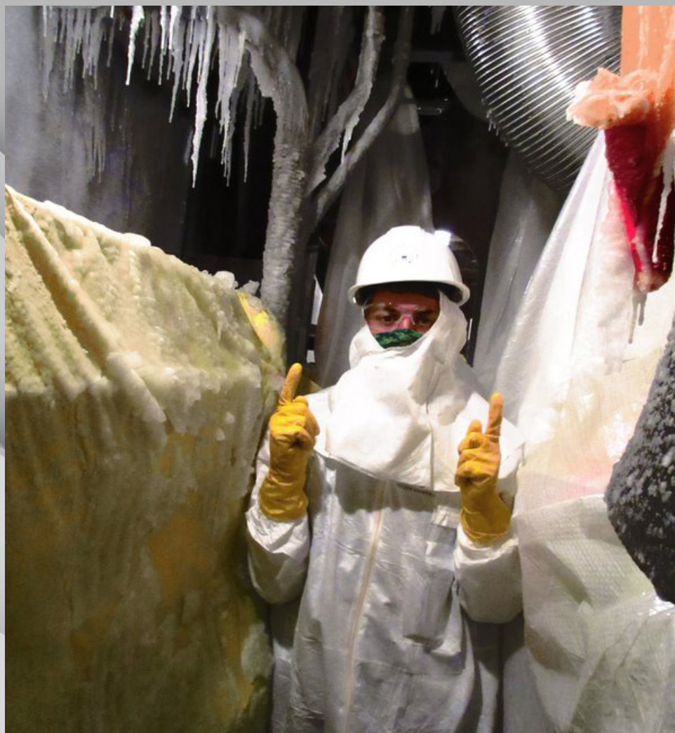
Nuclear Regulator Apprenticeship Network participant Hayden Page visits the plant's condenser containment system at the Sequoyah nuclear power plant in Tennessee.
