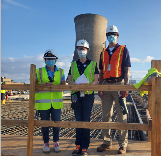
NRC inspectors (left to right) Katherine Warner, Liz Andrews and Mark Henrion observe workers preparing and pouring concrete for a dry cask storage pad on the Three Mile Island plant site in Pennsylvania.
