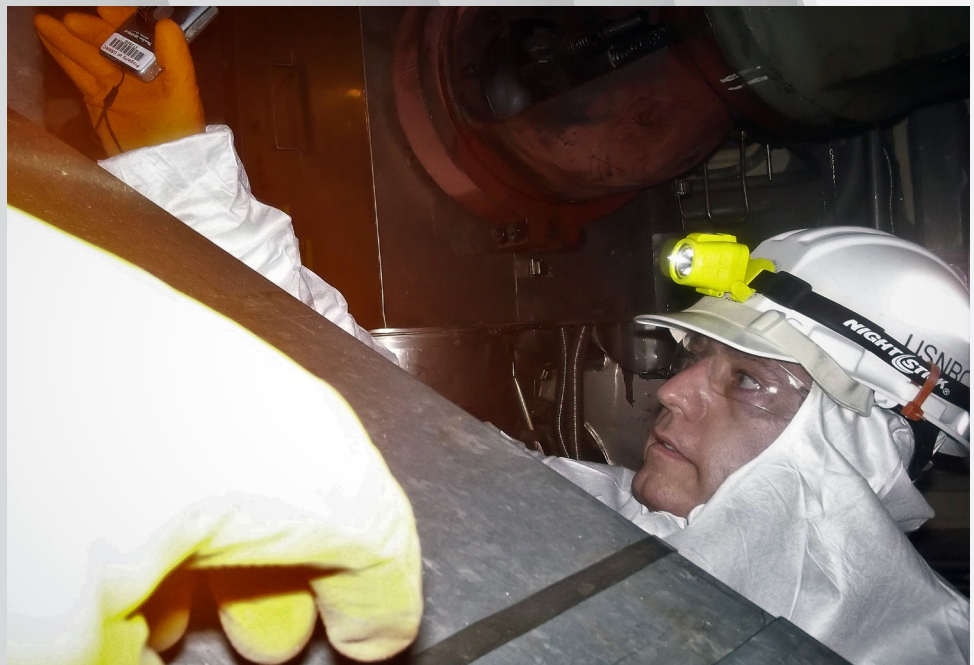
At the Susquehanna Unit 1 nuclear power plant, Senior Resident Inspector Chris Highley enters the Pennsylvania facility's containment during a refueling and maintenance outage to evaluate material conditions in this protective structure that surrounds the reactor.
