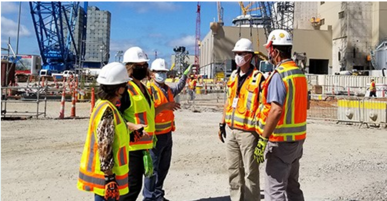
At Vogtle construction site: Laura Dudes - Region II Regional Administrator, Marissa Bailey - Division Director for Division of Construction Oversight, Brian Kemker - Vogtle Senior Resident Inspector, Jason Eargle - Vogtle Senior Resident Inspector, and Raju Patel - Reactor Operations Engineer
