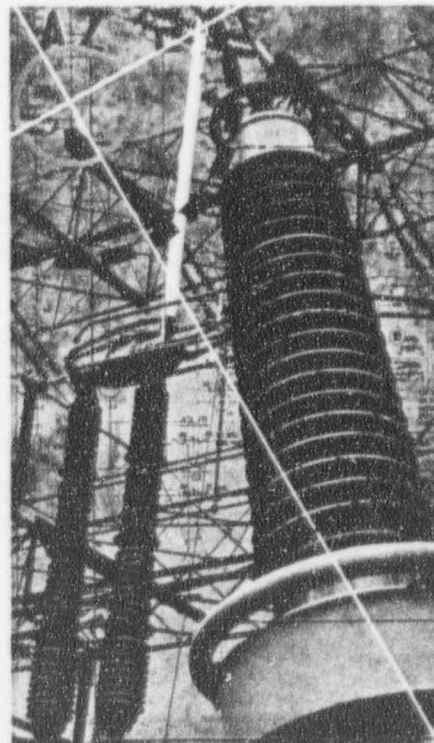
Substation insulators symbolize the underlying strength of our Core Electric Business.
