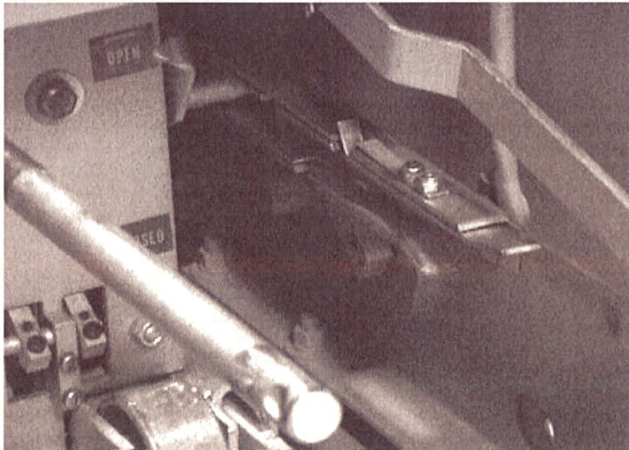
Breaker Closing and Trip Linkages. (Both shown down)
