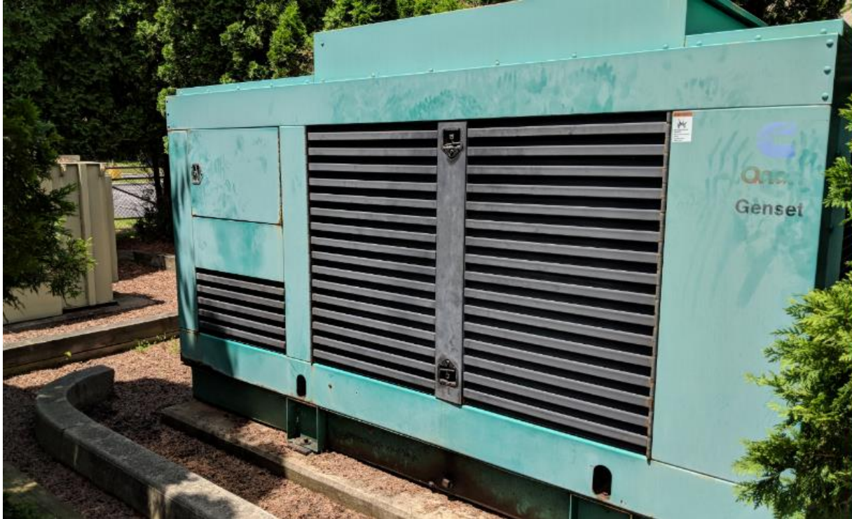
Coatesville EOF Emergency Diesel
