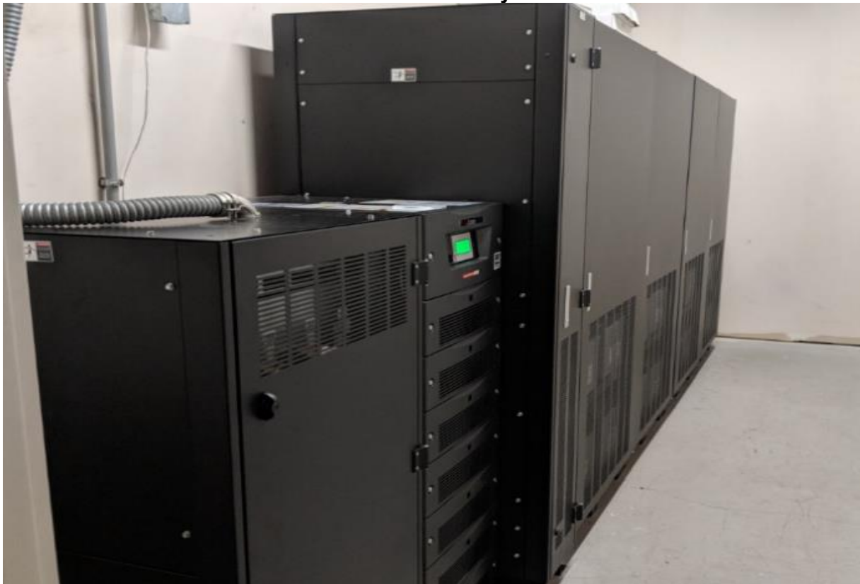
Coatesville EOF Battery Room
