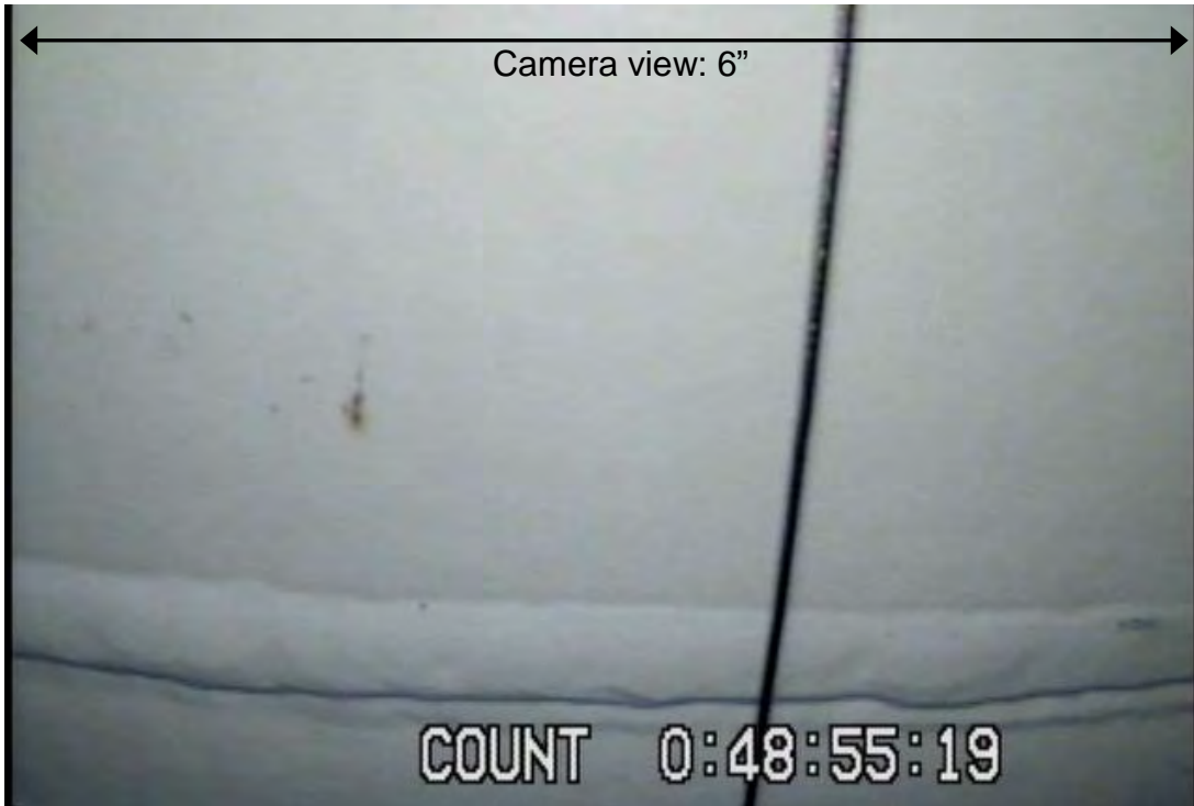
28. Scan 28 slight rust discoloration
