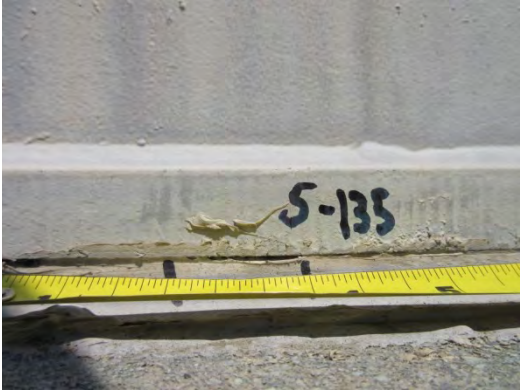
7. Cell 5 Caulking As-Found
