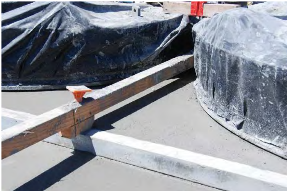
4. Photo taken during HB ISFSI concrete placement showing a construction aid most likely used to keep steel angles from moving during construction
