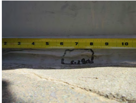
14. Cell 5 Caulking As-Found
