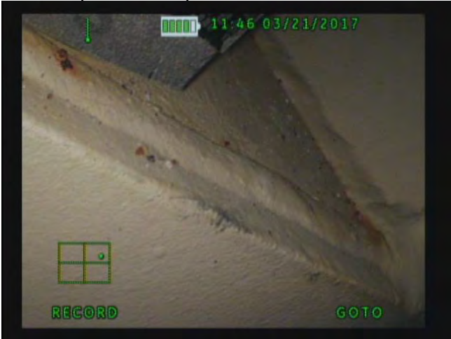
19. Overpack, rust spots
