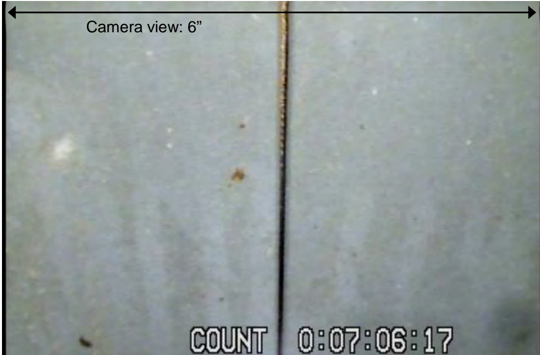
56. Scan 6 rust spots
