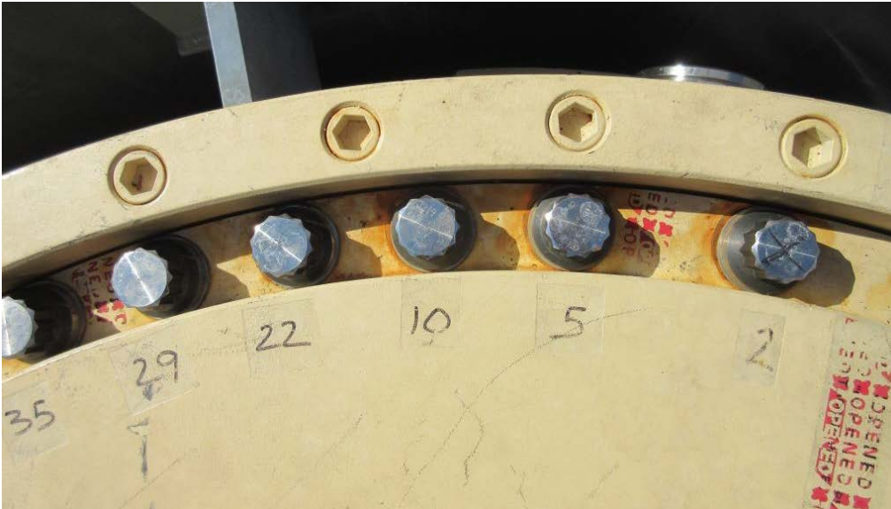
15. Rust staining around overpack lid closure bolting
