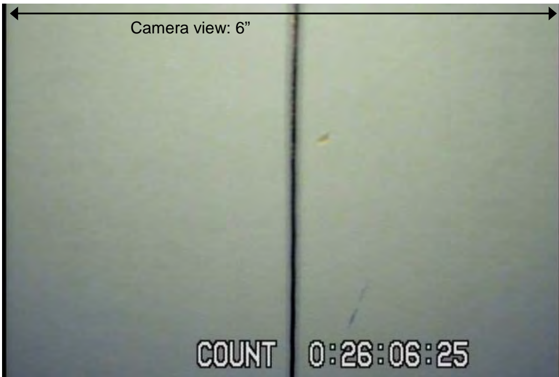
35. Scan 55 slight rust discoloration
