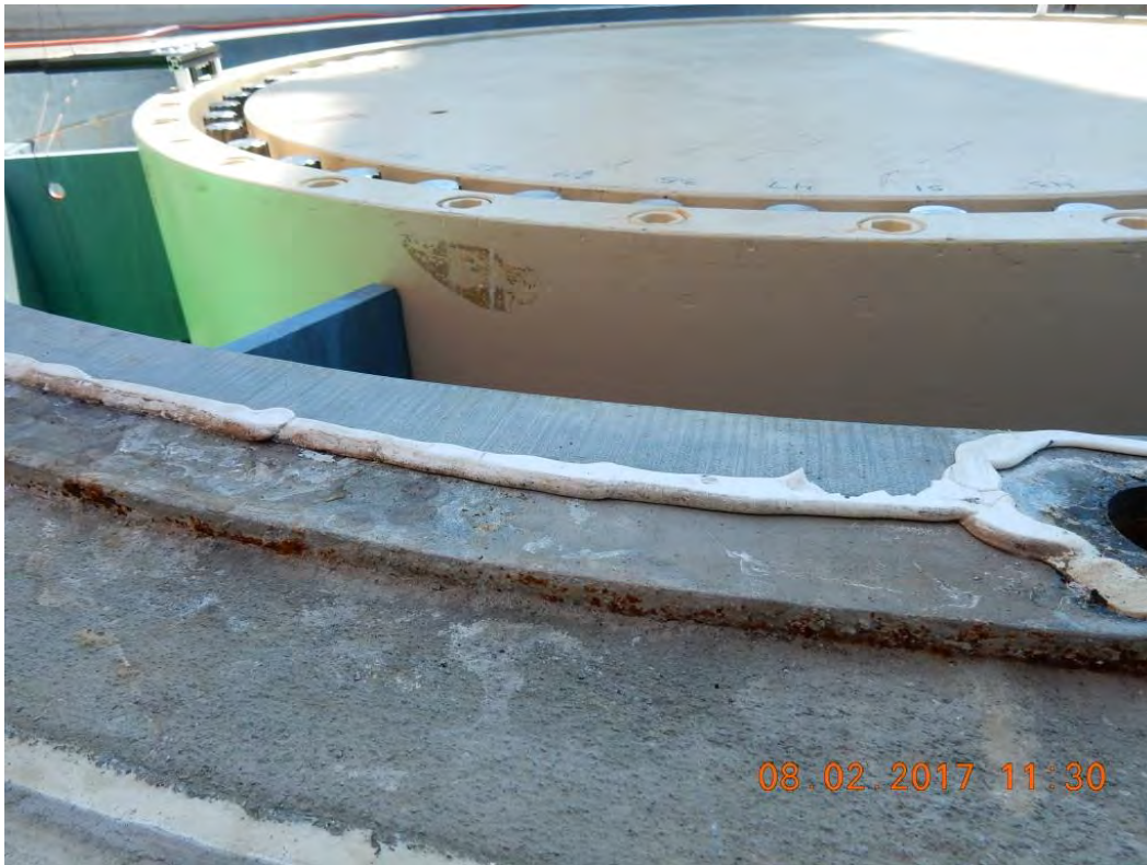
48. Rust at vault lid ring to concrete interface
