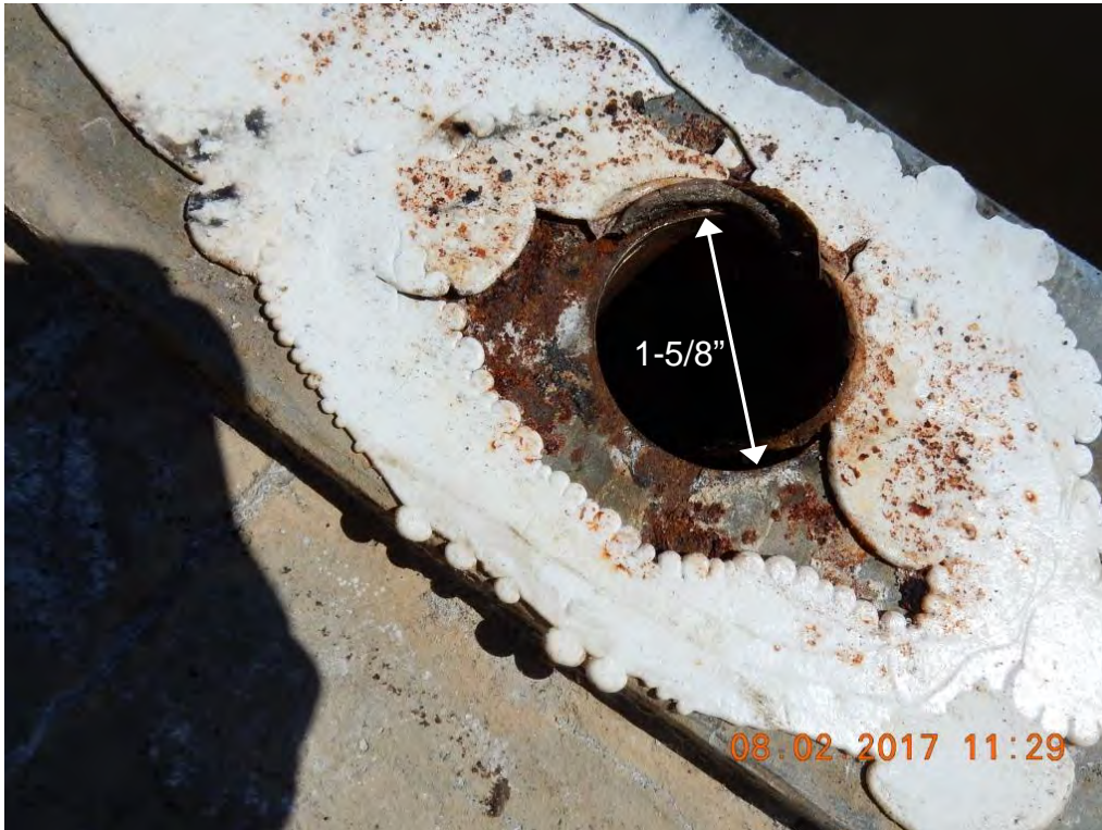
46. Vault lid ring bolt hole #3 corrosion products
