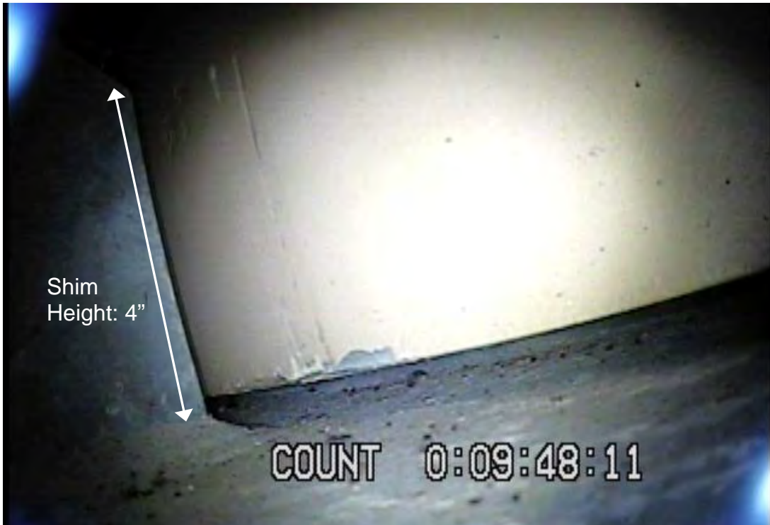
42. Overpack south east section coating scrape adjacent to seismic shim
