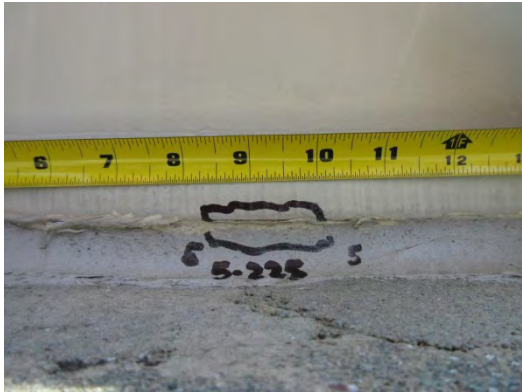
13. Cell 5 Caulking As-Found
