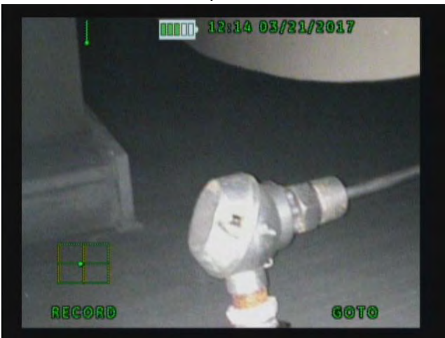
3. Vault Liner and Temperature Probe
