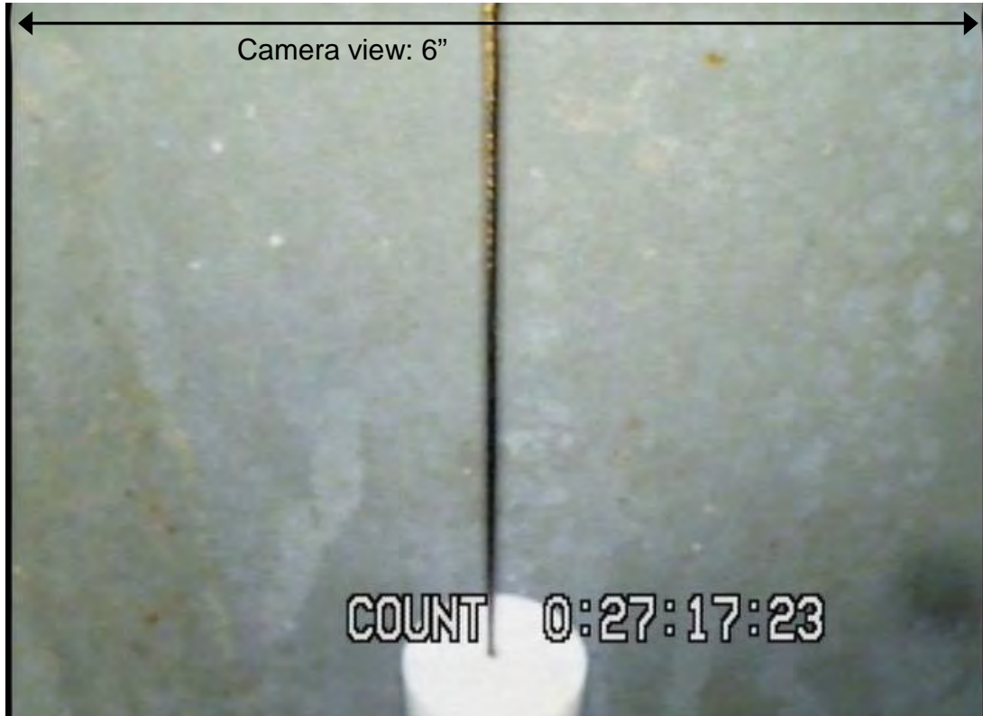
59. Scan 16 rust spot
