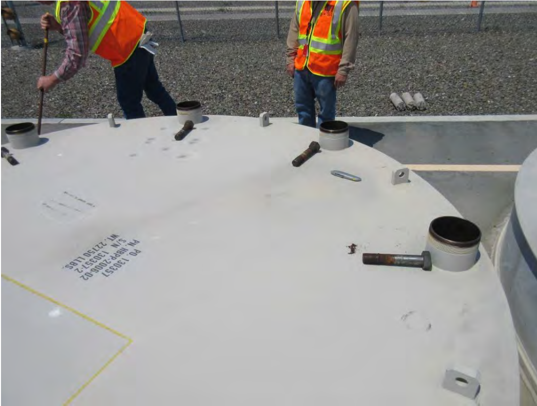
62. Removed hold down bolts lying adjacent to bolt ports
