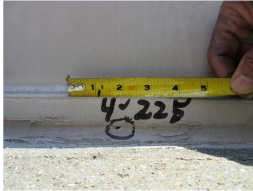
4. Cell 4 Caulking As-Found
