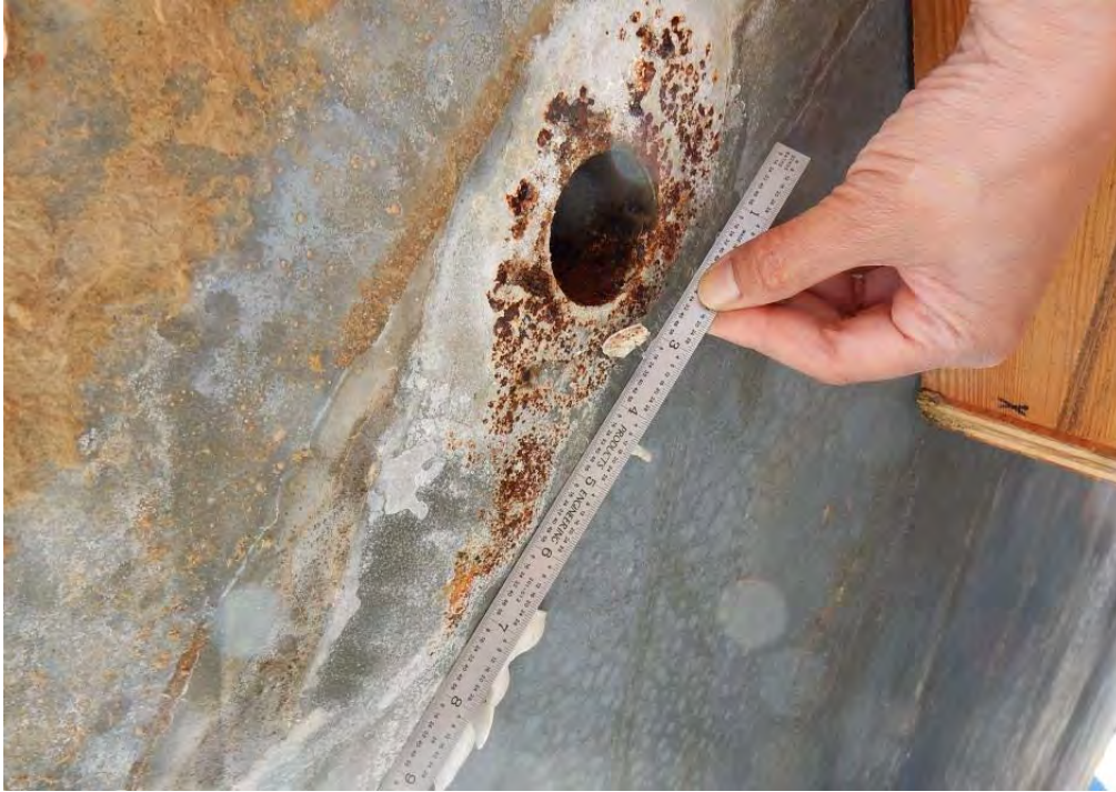
7. Underside hole #3 showing corrosion prior to cleaning
