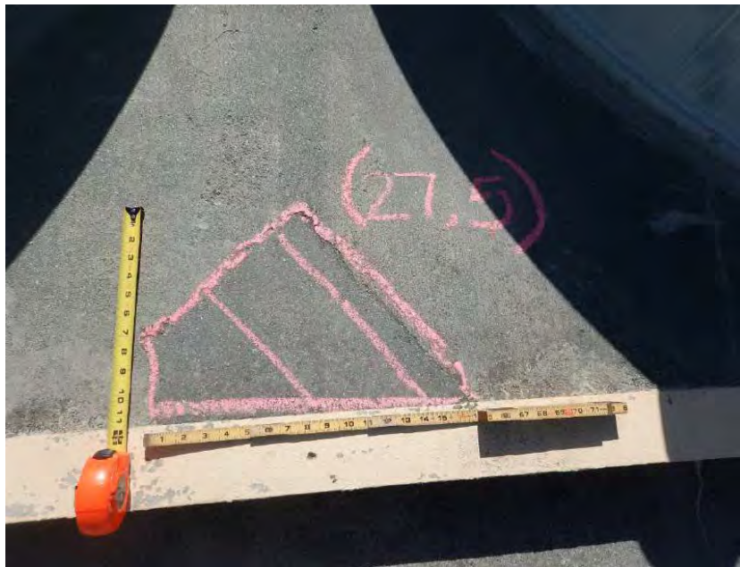
2. Center disbanded patch at (27, 5) that is approximately 17" by 11"
