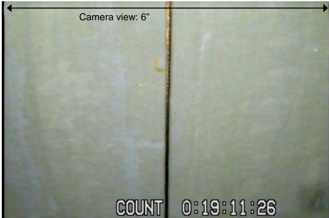
58. Scan 10 rust spot
