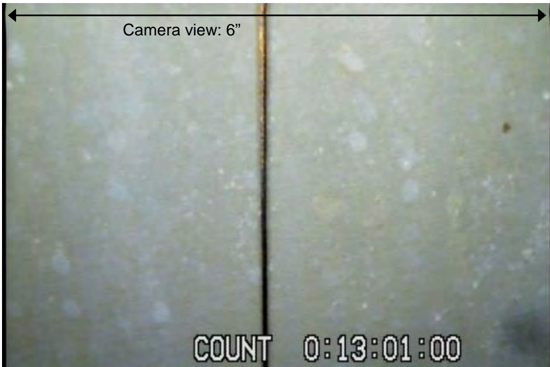
57. Scan 8 rust spot
