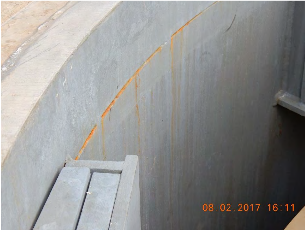
49. Rust staining at vault lid ring to vault liner interface
