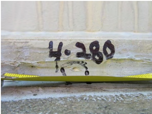
5. Cell 4 Caulking As-Found
