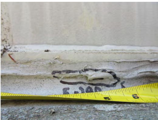
11. Cell 5 Caulking As-Found
