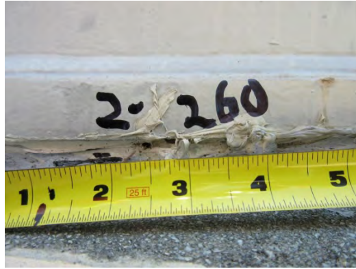
2. Cell 2 Caulking As-Found
