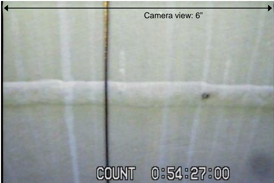
60. Scan 38 Dark spot – possible coating damage – no rust discoloration
