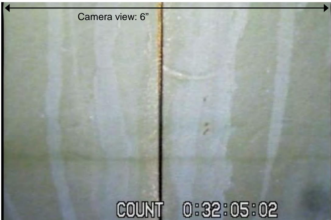
61. Scan 76 rust spots
