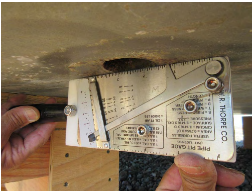
12. Measuring pit depth <math><1/16\text{''}</math>
