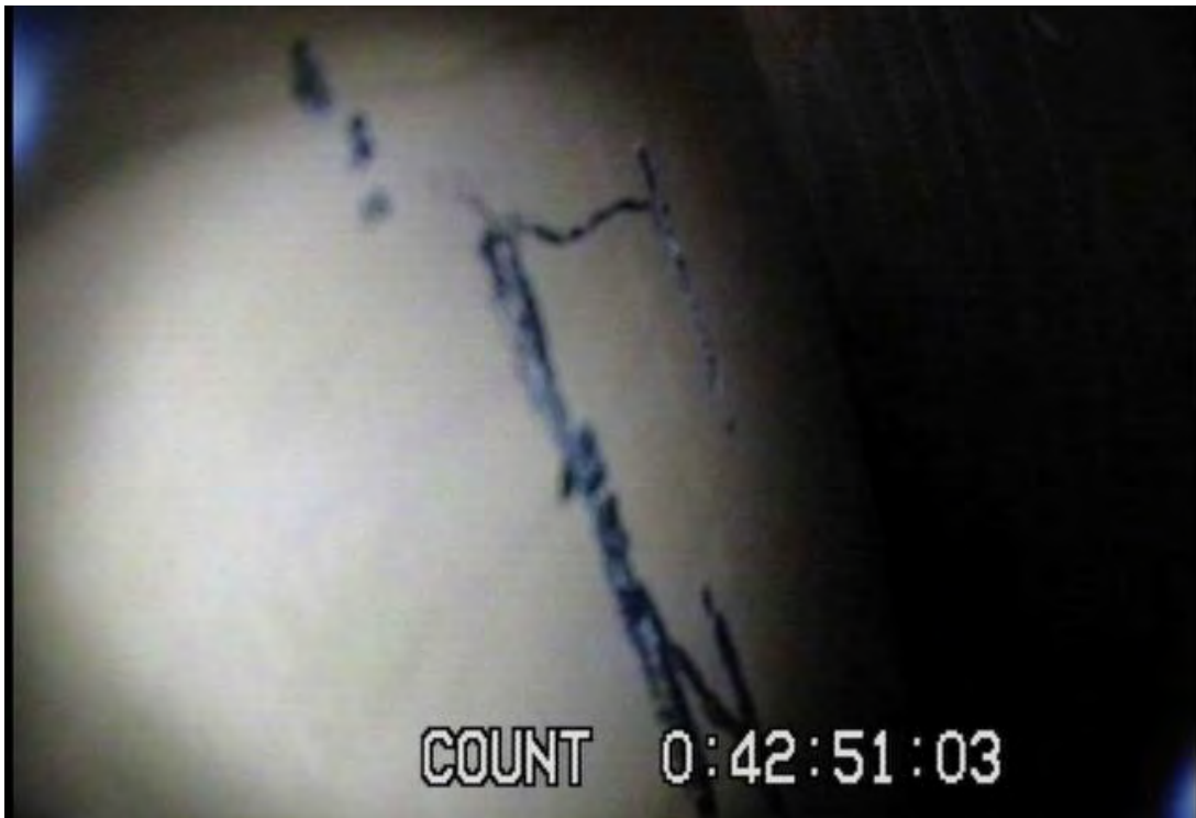
39. Scan 1 / Scan 80 area coating scrape
