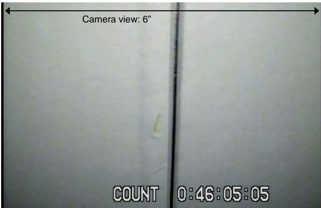
27. Scan 26 coating chip with slight rust discoloration
