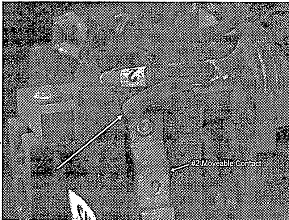
Figure 1 Wire Interference With Alternate Feeder Breaker Position Switch Moveable Contact
