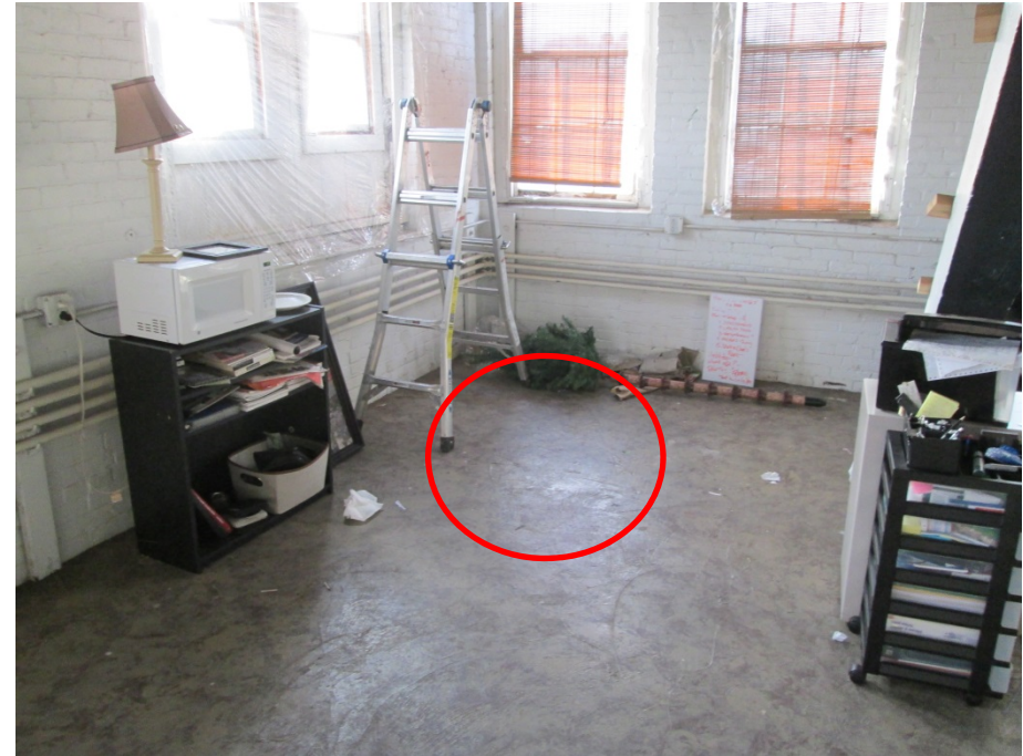
A-2. Area of Contamination Identified on the Third Floor of Building D (photo looking approximately southwest)
