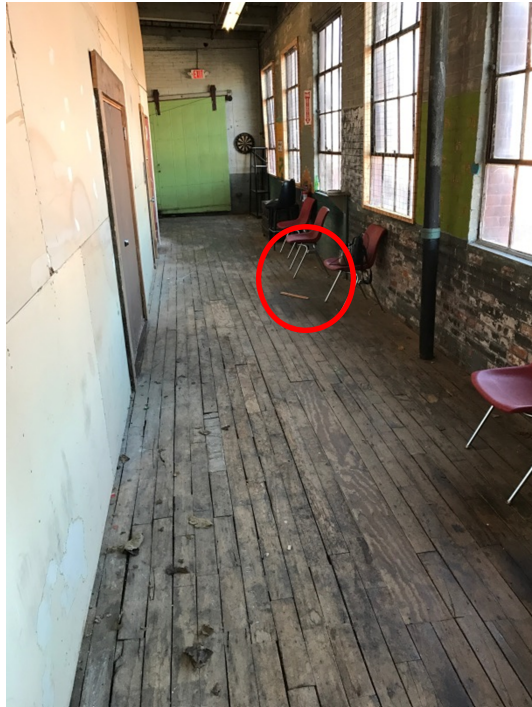
A-1. Highest Gamma Response Located on the Fourth Floor of Building B (photo looking approximately east)
