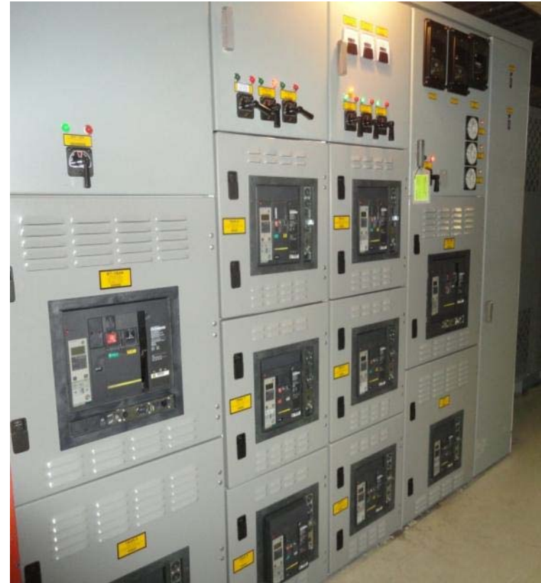
Restored Switchgear 1B4A
