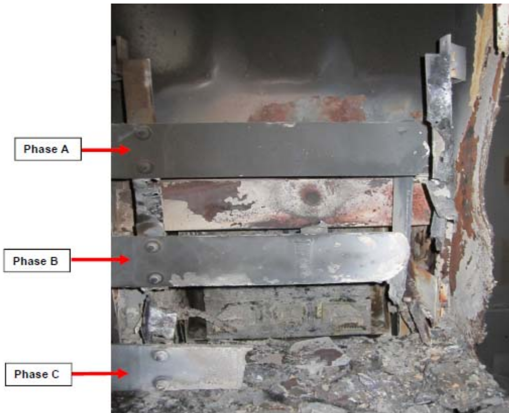
Damaged 1B4A Cubicle
