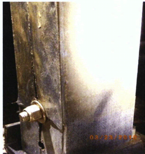
Photo 5 – Failed pipe column at FRP bearing pad
