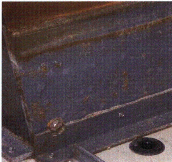
Photo 14 – Blistered Pipe Saddle Side Plate
