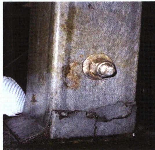
Photo 2 – Failed 3-1/2" pipe column with bottom shearing and mushrooming
