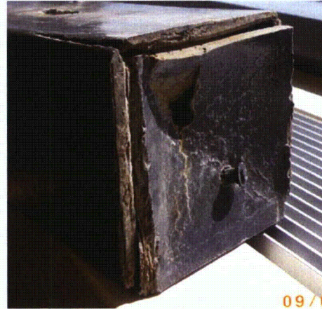
Photo 12 – Bottom view of failed pipe column & pad pushed into column
