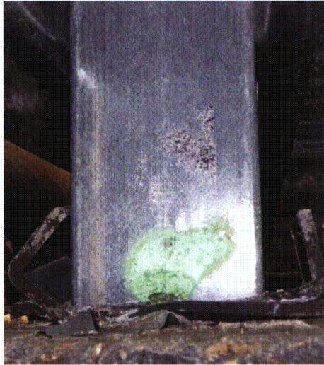
Photo 11 – Failed FRP bearing pad under pipe column
