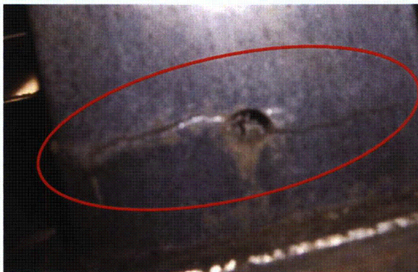
Photo 4 – Pipe column starting to shear along face
