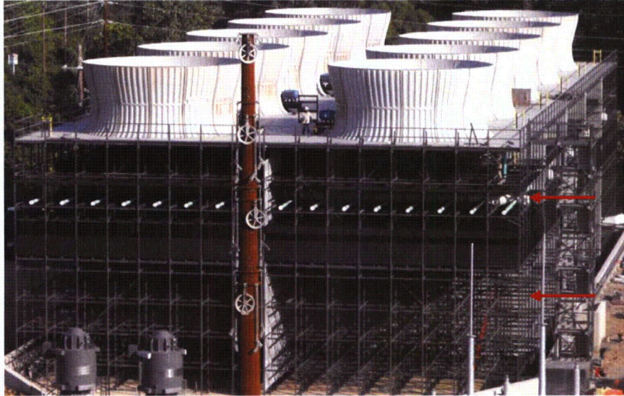
Photo 8 – Photo of counter-flow tower with column splice elevations shown by red arrows.
