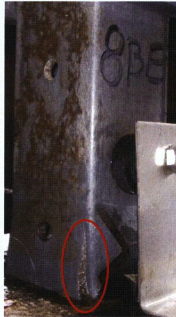
Photo 7 – Cracked 3-1/2" pipe column at corner
