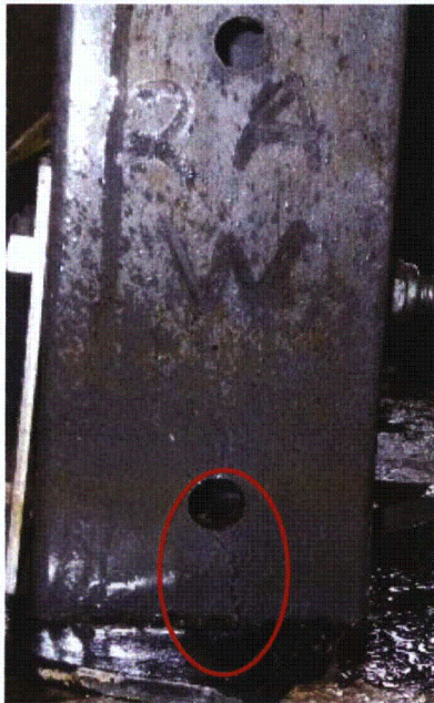
Photo 6 – Cracked 3-1/2" pipe column under a bolt hole
