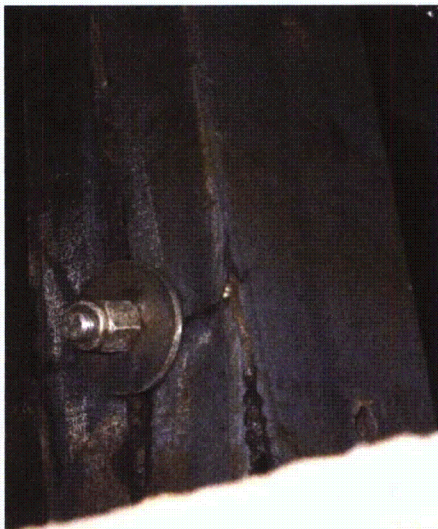
Photo 1 – Over tightened bolt at failed 3-1/2" pipe column
