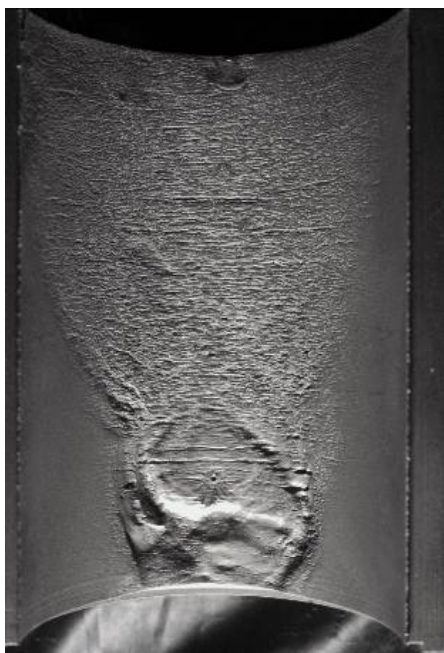
Example of Sectioned CRDM Nozzle Mockup Volumetric Leak Rate = 0.1 gpm Volumetric Wastage Rate = 4.1 in 3 /yr
