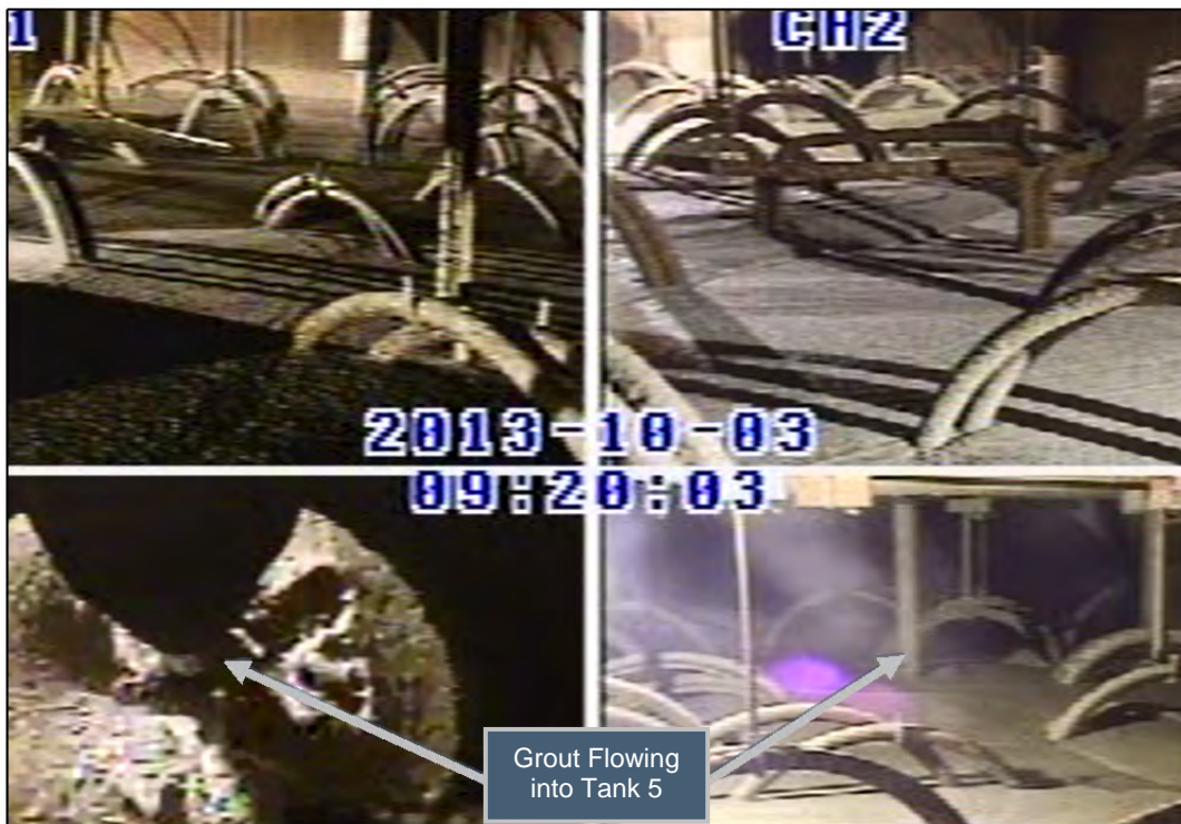
Figure 3.2-3: Bulk Fill Grout in Tank 5 during the Filling Process (Lift 8) Simultaneous Camera Views from Four Risers
