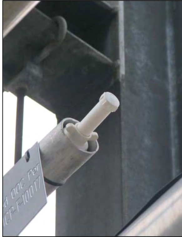
Figure 3.1-1: Tank 5 Bearing Water Supply Pipe Isolated (Tank 5)
