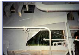
Fig. 2: Remote cooling tower sump
