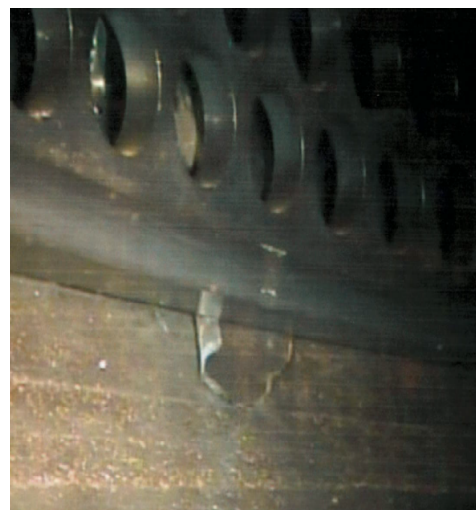
View of the impeller piece looking up from below the flow skirt.
