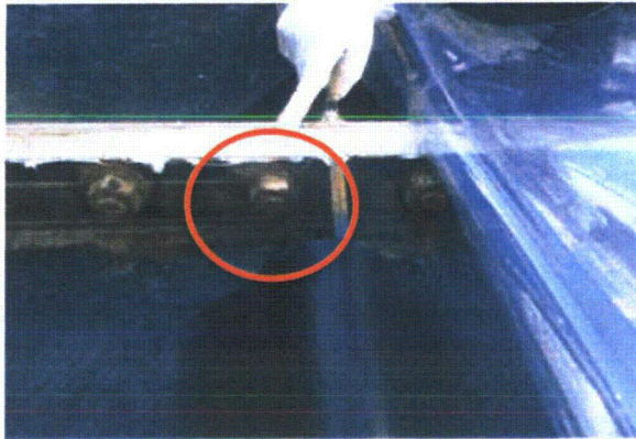
A loose blot at a flange part of the bottom plate (Photographed on September 19, 2013)
