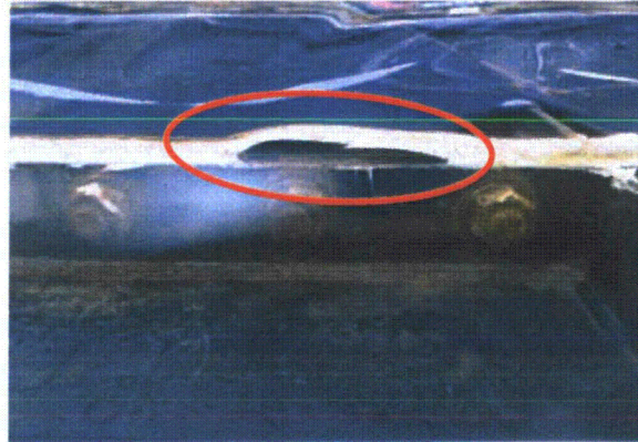
Swelling of the sealing material at a bottom plate flange part (Photographed on September 19, 2013)
