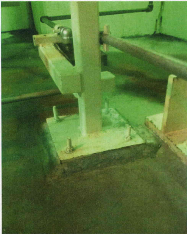
Photo 1 Anchor Threading Substantially Past Nut
