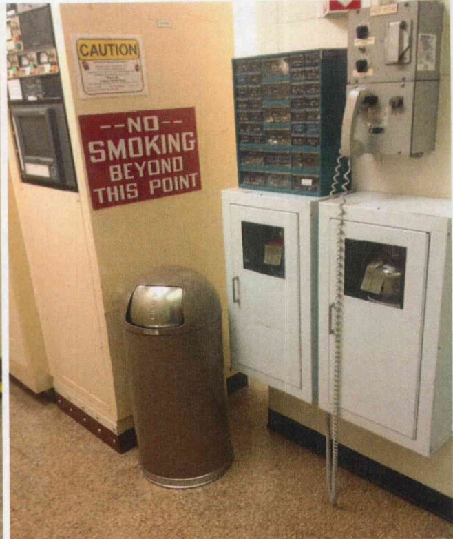
Photo 4 Unrestrained Trash Can and Light Bulb Storage
