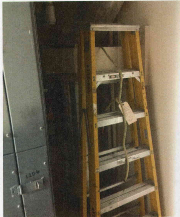
Photo 2 Ladder Loosely Tied Adjacent to MCC F11A
