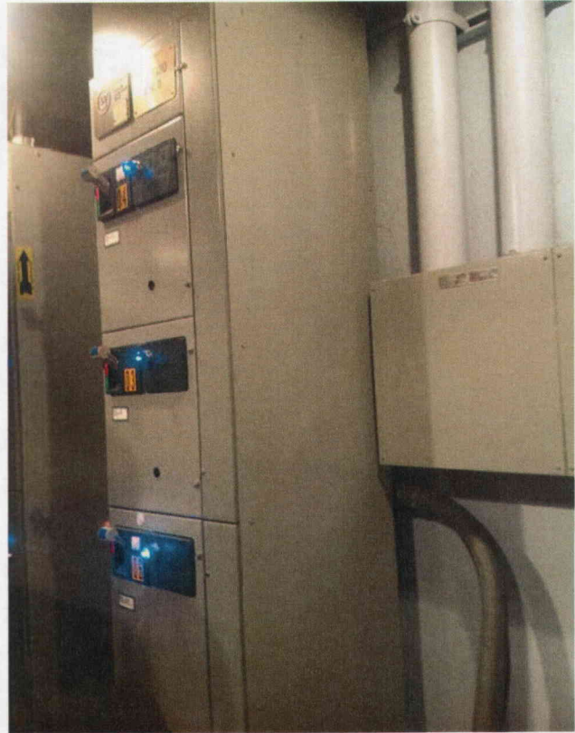
Photo 2 Movement of MCC Restrained by Adjacent Component
