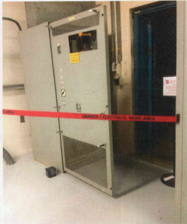
Photo 4 Cabinet DCB-2P Door Left Open
