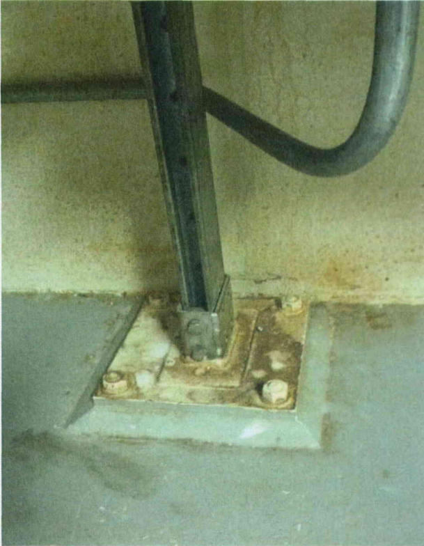
Photo 3 Minor Corrosion on Anchor Plate
