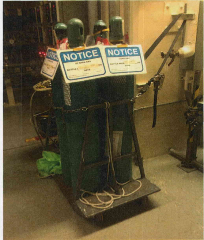
Photo 4 Cart Containing Gas Canisters Loosely Restrained
