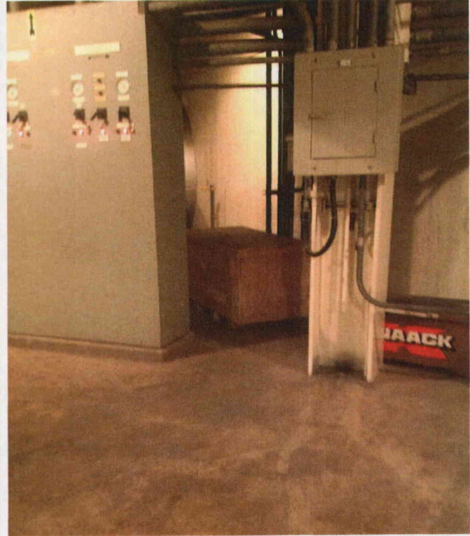
Photo 2 Unrestrained Storage Containers
