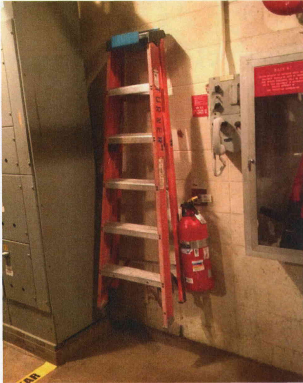
Photo 1 Fire Extinguisher not Restrained and Masonry Wall
