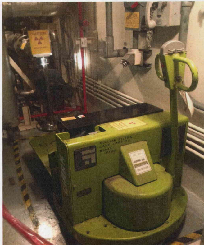
Photo 2 Nuclear Filter Cask Cart Not Restrained
