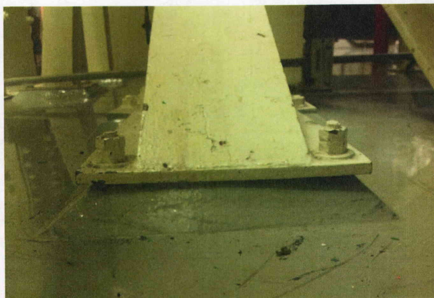
Photo 2 Gap Between Grout and Anchor Plate
