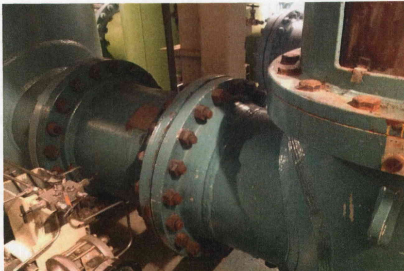
Photo 3 Minor Corrosion of Pump P3-2
