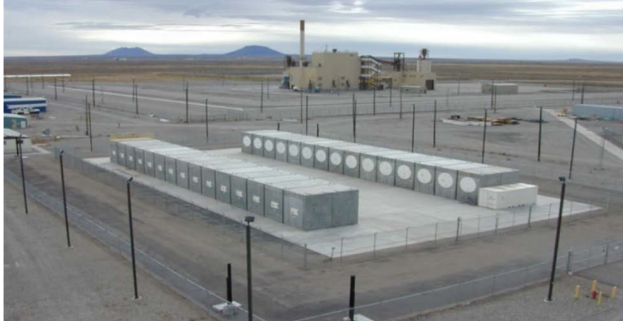
Figure 3.6. Photograph of a NUHOMS Storage Facility at INL (photograph courtesy of INL)
