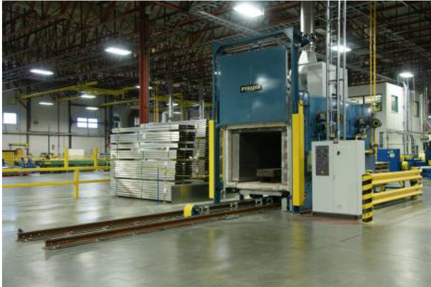
Flattening and/or heat treatment furnace
