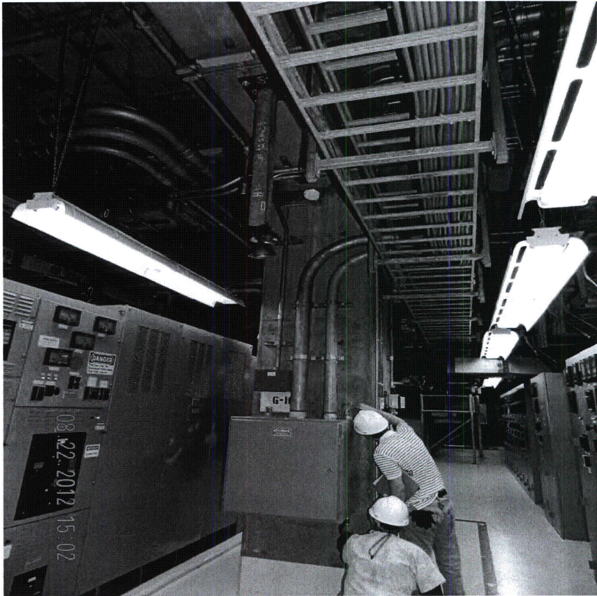
"Overhead Equipment or SSC"
