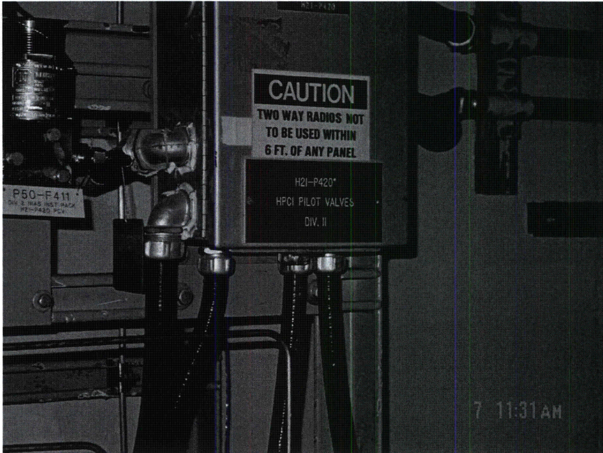
Attached Flexible Conduit Lines on Instrument Rack
