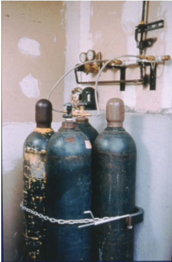
Oxygen Manifold System - Oxygen Supports Combustion
