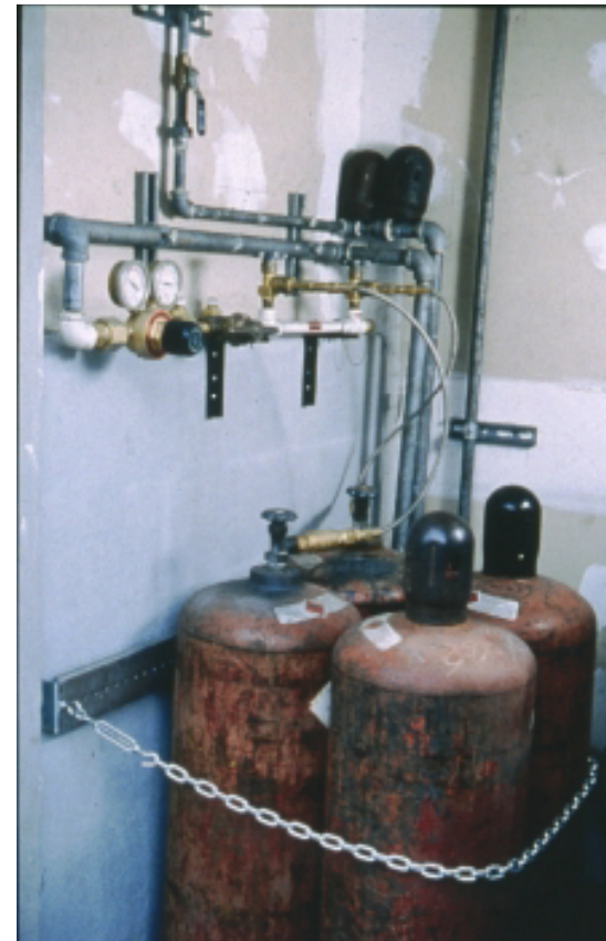
Acetylene Manifold System – A Fuel Gas
