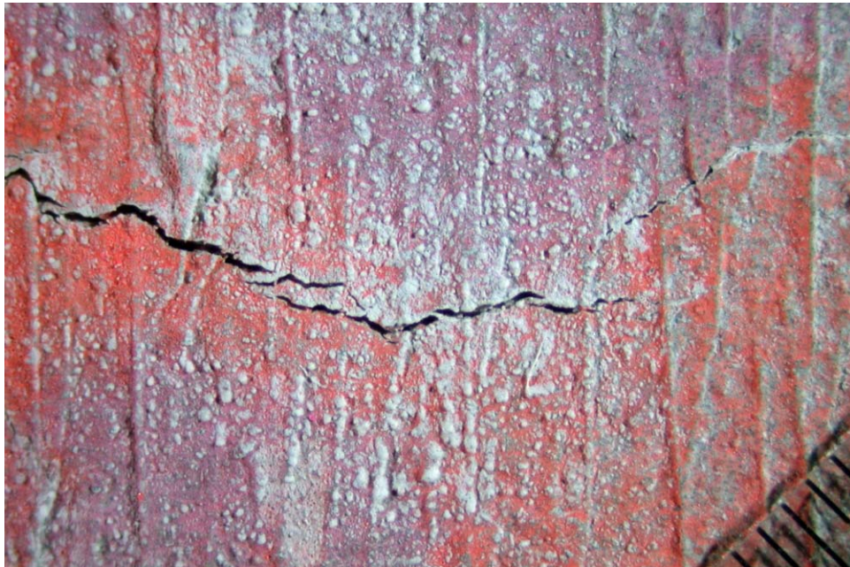
Fig. 3 Magnified view of crack on top surface of Core #4TP. Note discontinuous, tear-like appearance of crack.
