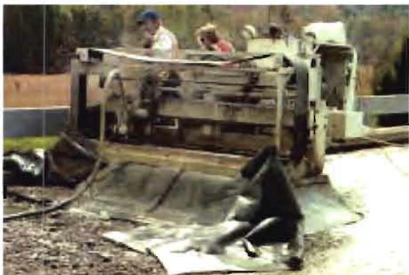
Figure 1: Hydro machine in action. (Note the rubble in front, compared to the milled deck behind.)
