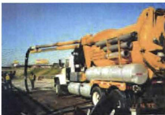
Figure 4: Vacuum truck with hose on boom; can stay off rebar mat but is slower picking up debris.
