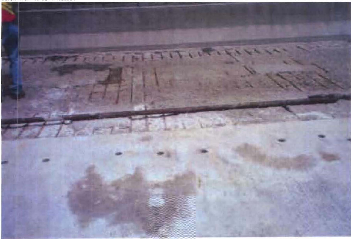
Figure 6: Finished hydrodemolition of half (background) of Bridge A0174 E. In the foreground, new latex modified concrete overlay. Note: 2" core holes in the overlay are where pull-off tests for direct tension were taken.
