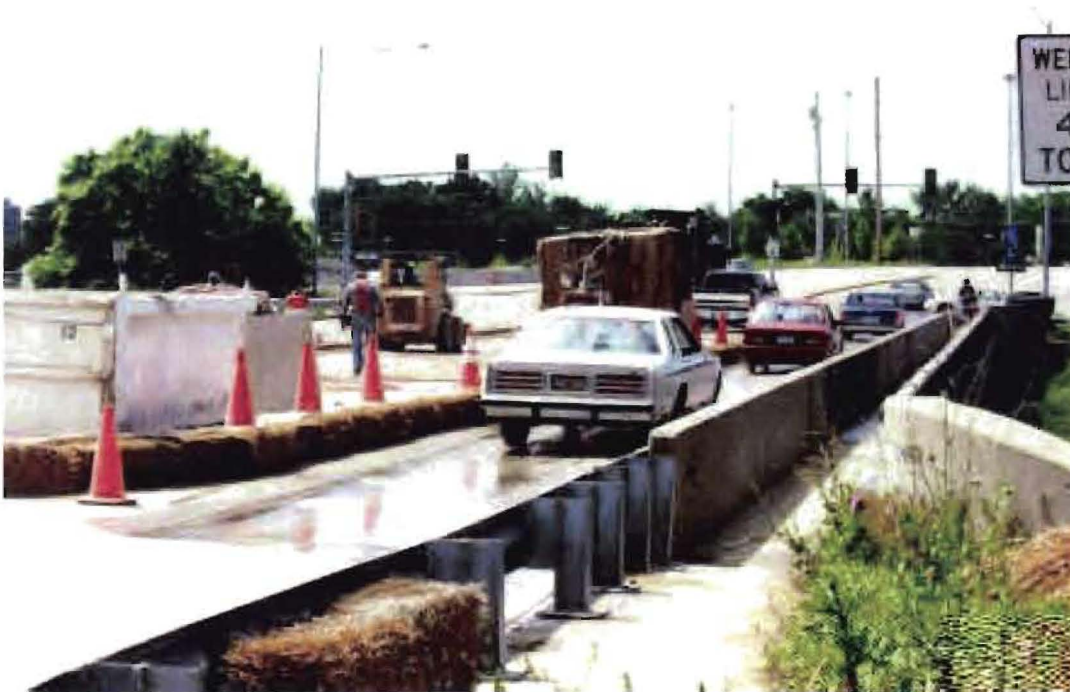
Figure 5: Shows traffic control and containment of blast water while hydroblasting for patches in two center lanes of a four lane bridge.
