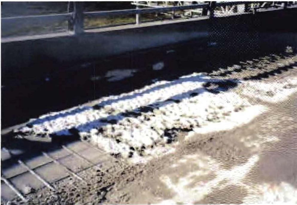
Figure 7: Poor concrete and a thin 6 1/2" upper deck made it necessary to do hydrodemolition at 13,000 psi . This is after the first pass (Note how clean the re-steel is in the foreground on the left). A second pass with the hydro-blaster was necessary to remove the island of unsound concrete left over the rebar in the center of the photo.
