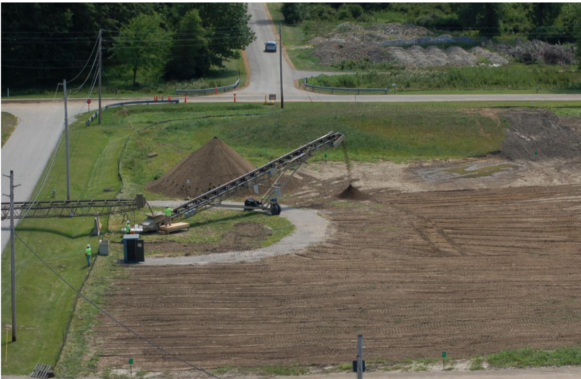
Exhibit 13, ScanSort System Clean Discharge (August 2009) (View from Radar Tower - Line 2 Road on the left and Pentolite Road at the rear)
