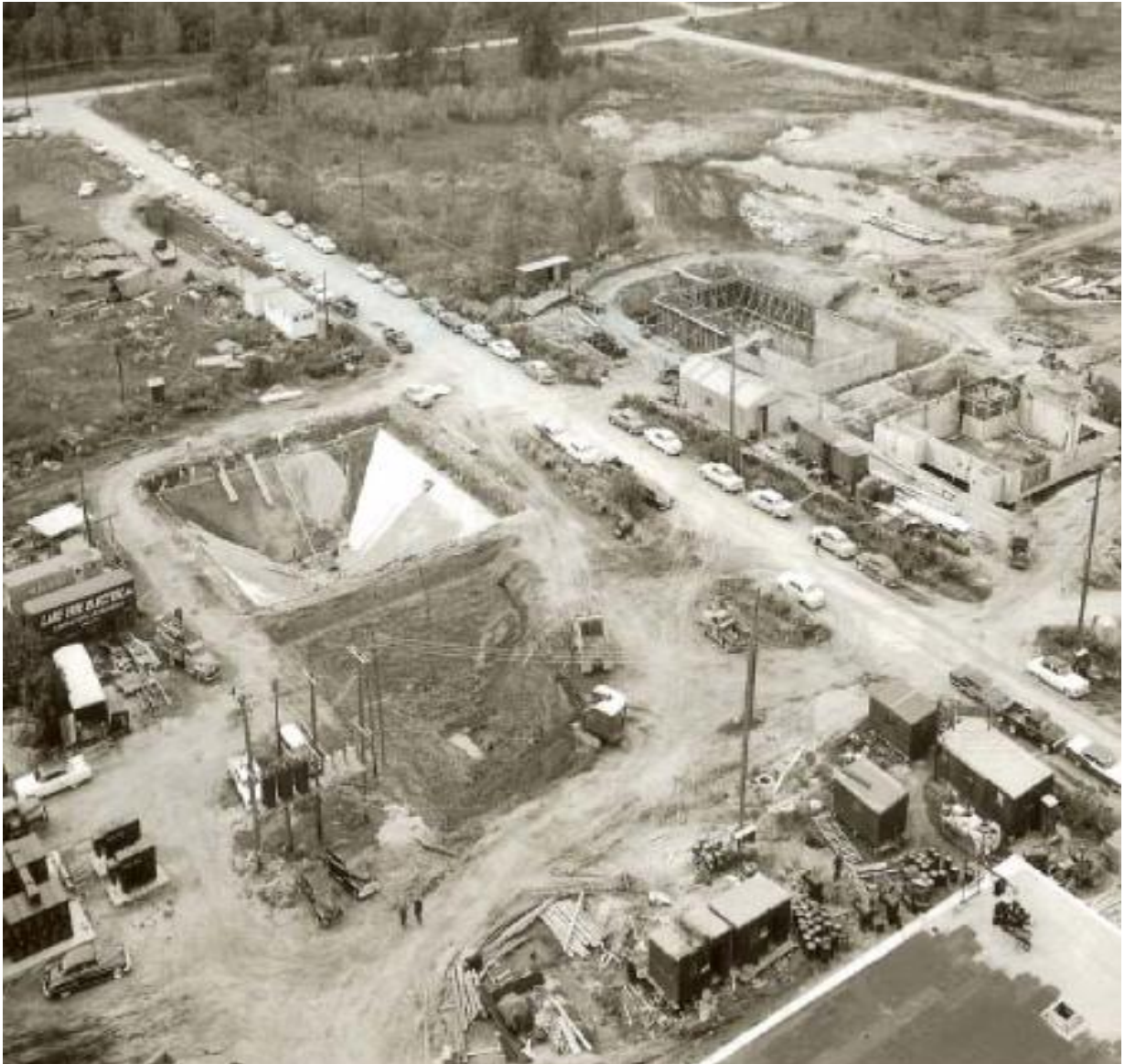
Exhibit 3, PBRF Construction Photo showing CRB Excavation in foreground (Aerial view from NE – Line 3 Road is in the center, Photo circa 1957)
