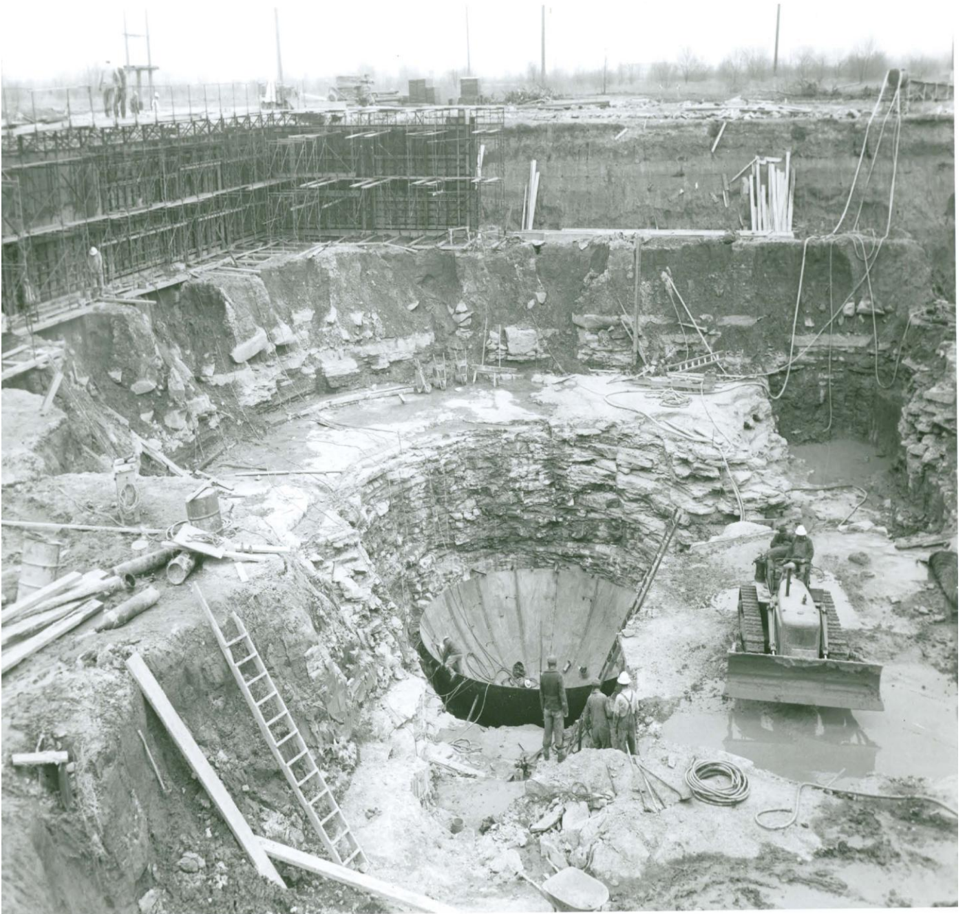
Exhibit 2, Construction Photo Showing Excavation for Reactor Vessel Foundation (Vessel foundation bottom liner is 59 feet below grade level, Photo circa 1955-56)
