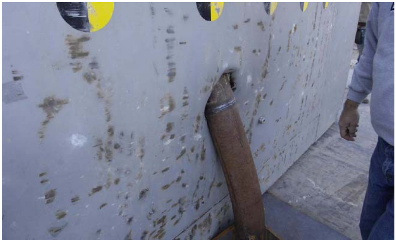
Figure 3.5-22 – LP1 Puncture Bar Damage before Removal of Bar
