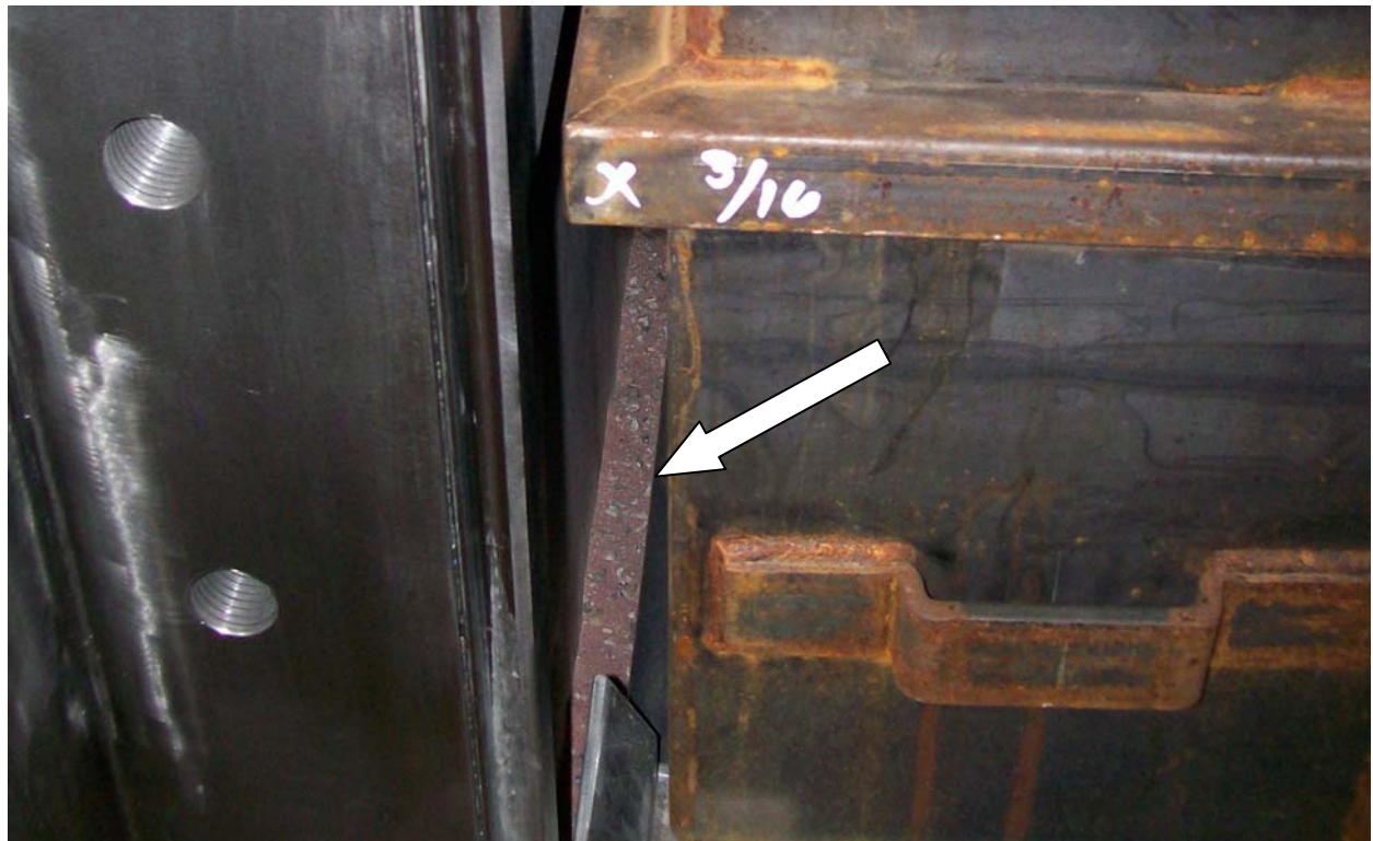
Figure 2.12.6-10 – Part of the Debris Between Roller Floor and Sidewall
