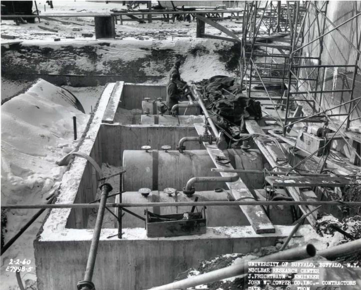
1960 construction photo showing the Tank Farm with the smaller tanks installed. All these tanks are currently in Wet Layup.
