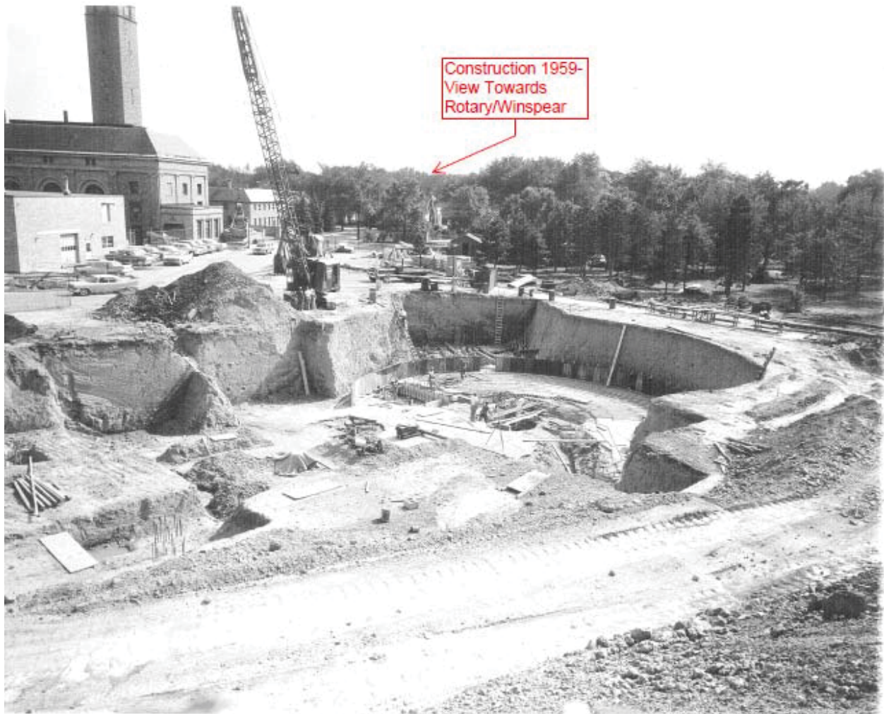
A Construction photo from 1959 showing the Primary Piping excavation into the bedrock in the foreground of the pit.
