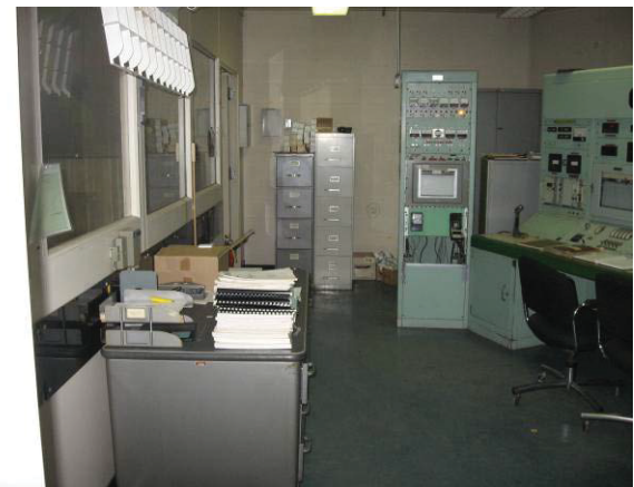
Photograph 36 Room 205 (Control Room)
