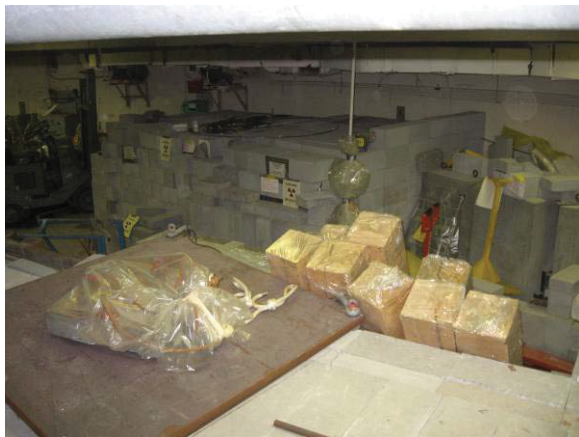
Photograph 66 High Radiation Area Neutron Level
