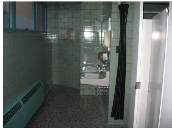
Photograph 6 Room 221 (Women's Restroom)
