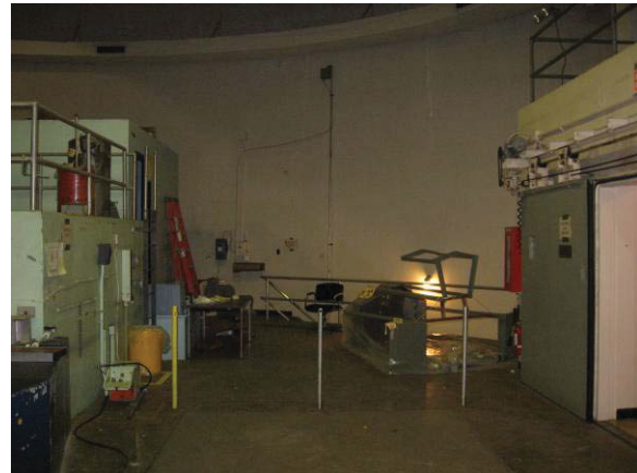
Photograph 42 Main Floor Control Deck
