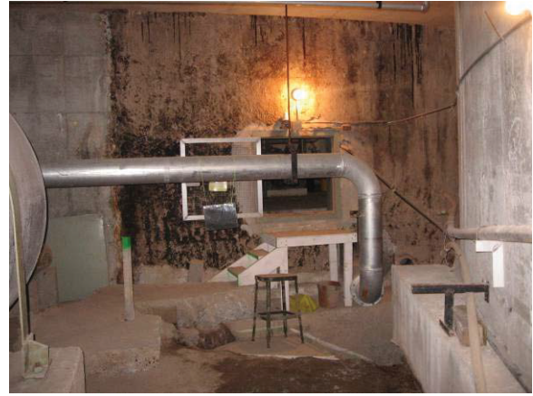
Photograph 31 N16 Tank Room
