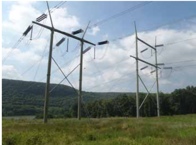
Photograph 1. Transmission Corridor in Area 13 East (Excess Cut Disposal Area), Facing Southwest
