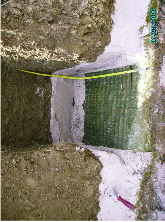
Fig. A.60. Close-up of vegetation barrier in AO2.
