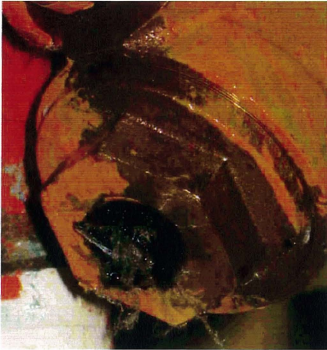
Figure 6 Failed plastic end cap on Dresden EDG 2/3 lube oil strainer
