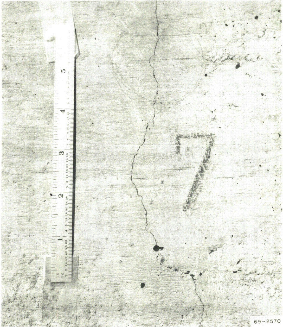
FIG. 84 TYPICAL CONCRETE CRACK.
