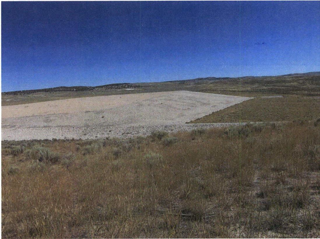
MAY 8/2011. PL-5. Eastern portion of the disposal cell; Diversion Channel No. 2 in foreground.
