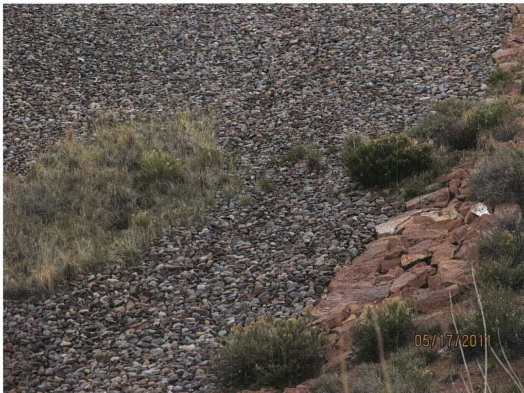
NAT 5/2011. PL-2. Vegetation in toe drain east of perimeter sign P-19.
