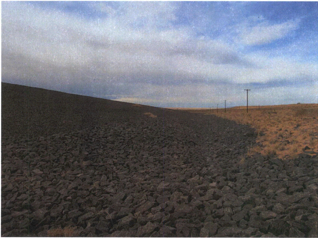
TUB 4/2011. PL-5. Northwest side slope and apron ditch of the disposal cell.
