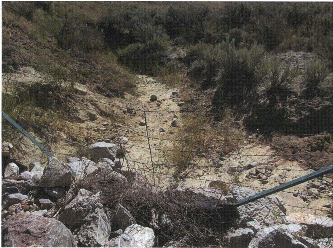
MAY 8/2011. PL-7. Exposed geo-fabric and erosion at the discharge point of Diversion Channel No. 1.
