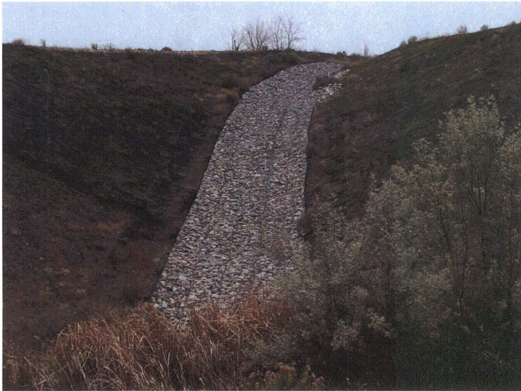
SHP 6/2011. PL-3. Outflow channel.
