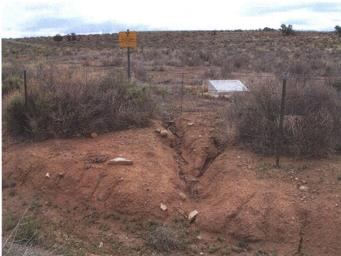
SRK 7/2011. PL- 1. Erosion under fence near site marker SMK-1.
