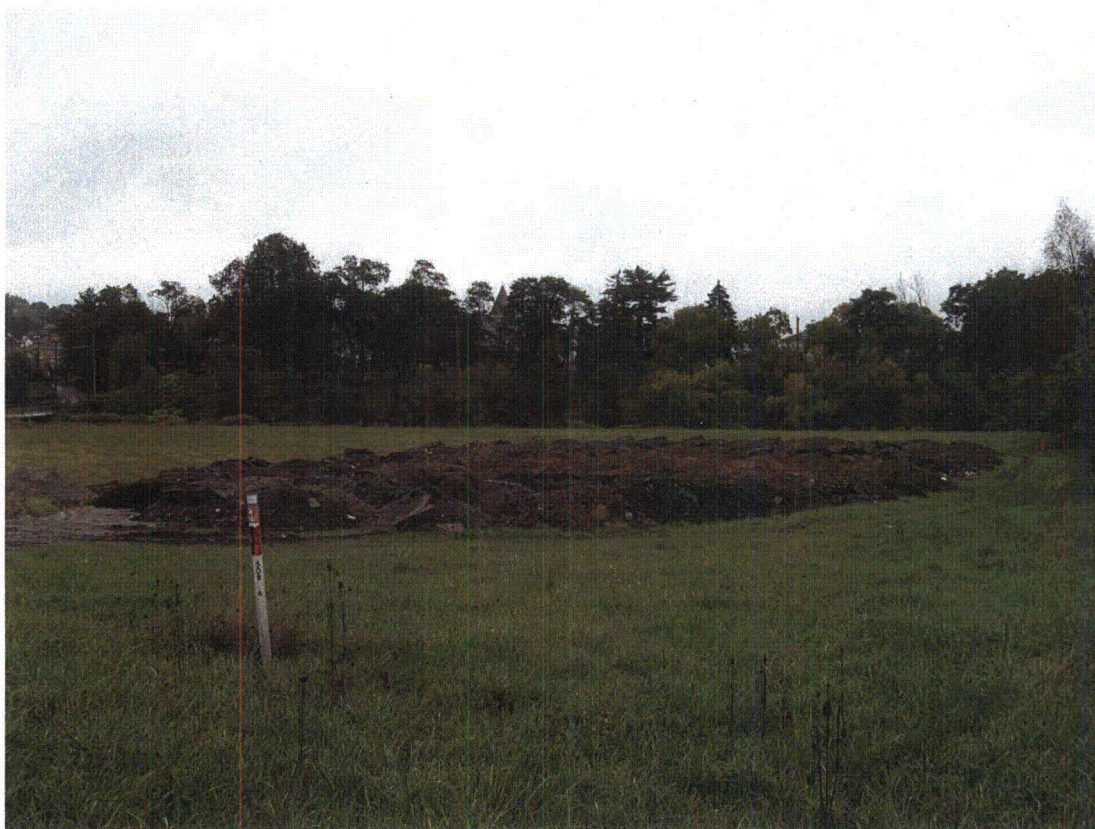
CAN 10/2011. PL-1. Fill material on Area C property.
