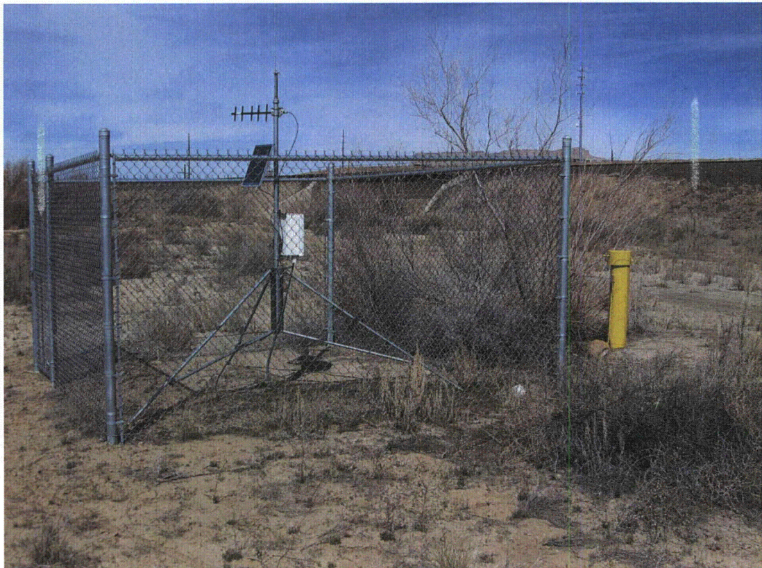
GRN 3/2011. PL-6. Monitoring well 0817 and enclosed telemetry tower.
