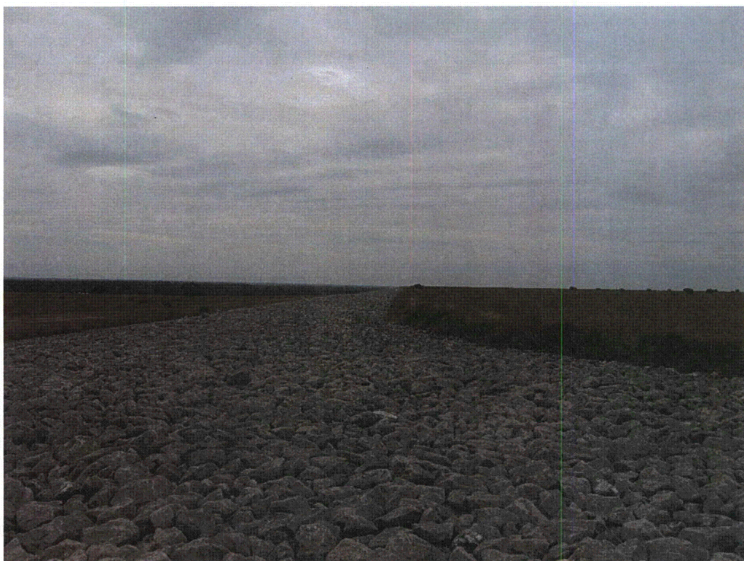
FCT 1/2011. PL-2. Contact between grass cover and riprap side slope of disposal cell, looking northeast down northwest side slope of disposal cell.
