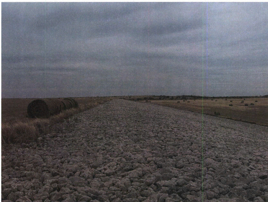
FCT 1/2011. PL-1. Contact between grassy top and riprap sides of disposal cell, looking down northwest face of disposal cell.
