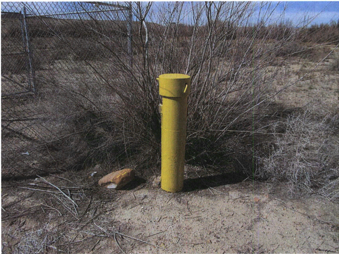
GRN 3/2011. PL-2. Monitoring well 0817.
