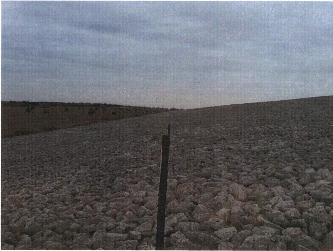
FCT 1/2011. PL-3. Looking down line of t-posts, south corner of disposal cell.
