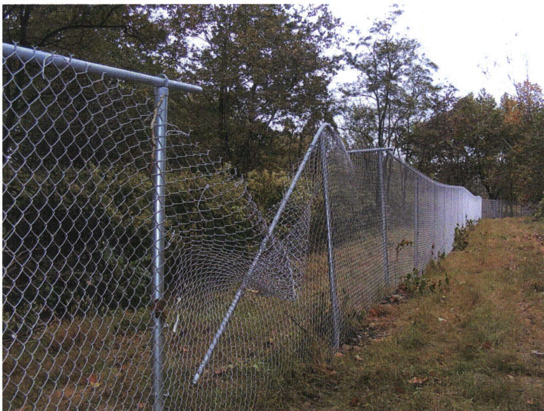
BUR 10/2011. PL-1. Damage to perimeter fence.
