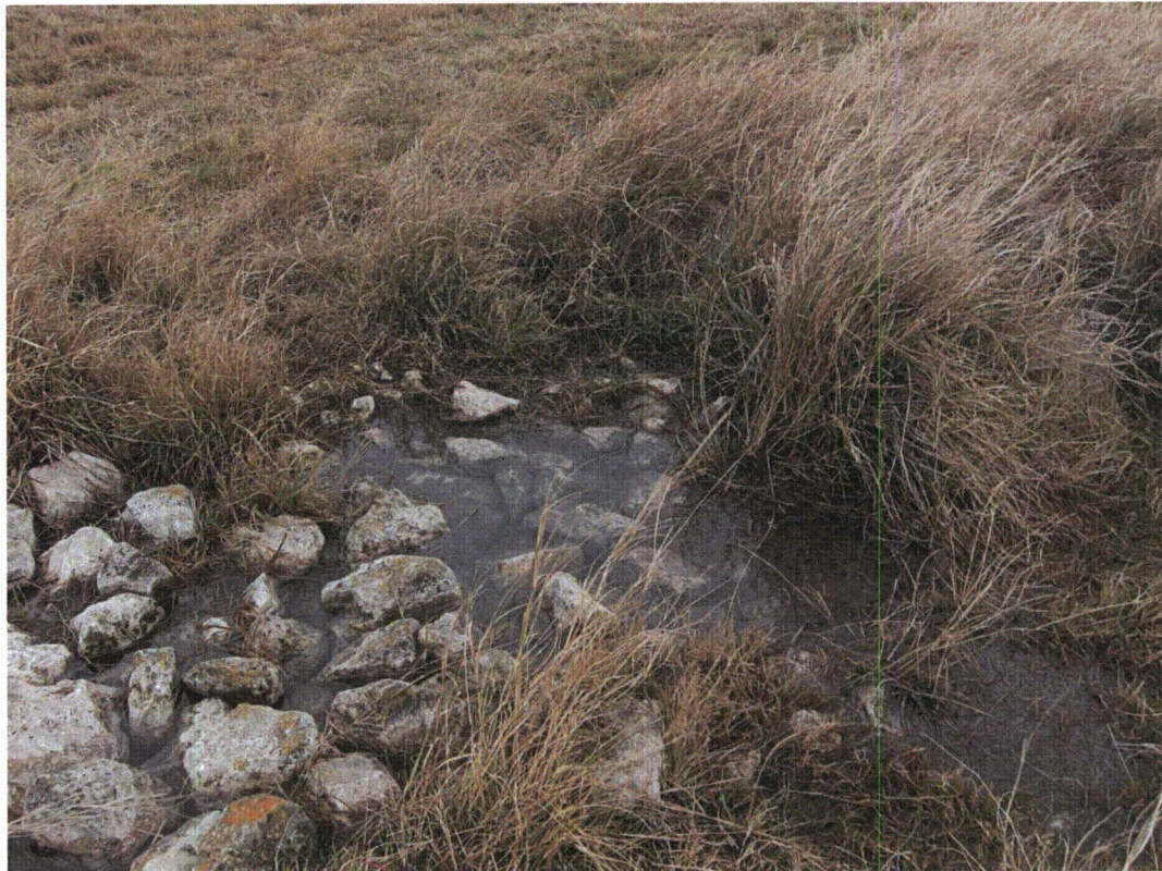
FCT 1/2011. PL-5. Water ponded at outlet of south rock drain.
