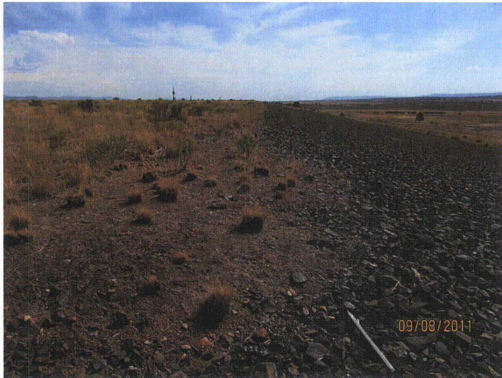
LKV 9/2011. PL-4. Photo taken (looking south) at intersection of west and north side slopes and top slope. Soil from top slope is being deposited onto side slope riprap.
