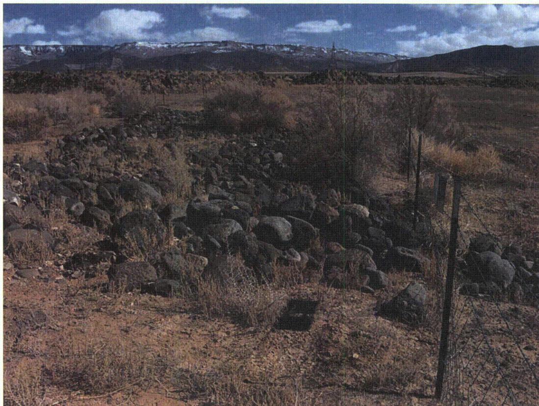
GRJ 3/2011. PL-4. Riprap erosion protection near the southeast corner of the perimeter fence.
