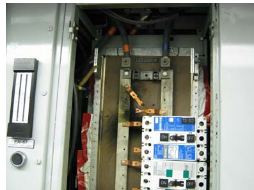
Figure 3-1: DC Panel ED-11-2 – After Fault Event
