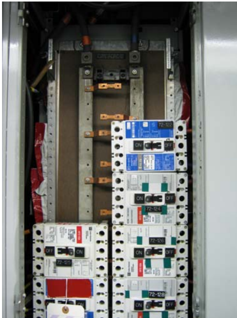
Figure 3-1: DC Panel ED-11-2 – Just Prior to Event
