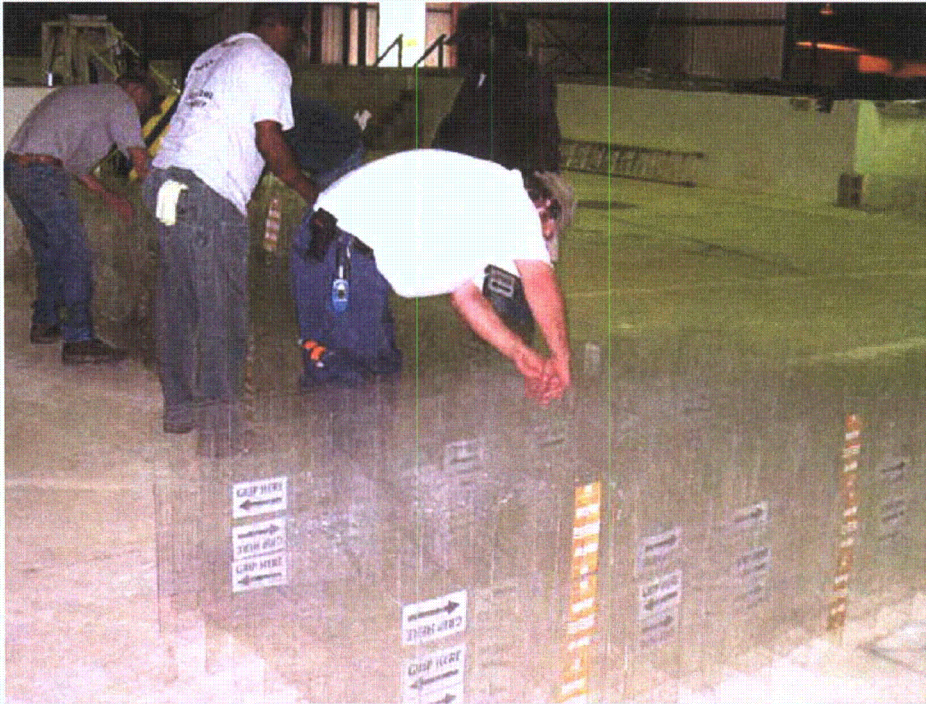
Figure 2-109. Third grid unit layer at right wall and center wall junction, viewed from pool side
