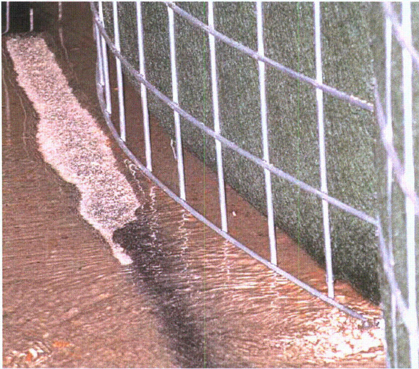
Figure 2-64. Close-up of seepage through vertical joint between units
