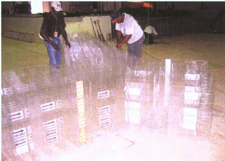
Figure 2-110. Top (fourth) grid layer installed along center wall/left wall buttress as viewed from pool side
