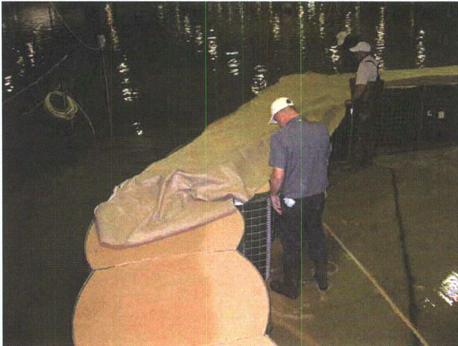
Figure 2-74. Covering top of wall with tarp to prevent further erosion
