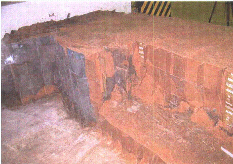
Figure 2-123. Right concrete wall abutment completed sand and mixture fill, viewed from pool side
