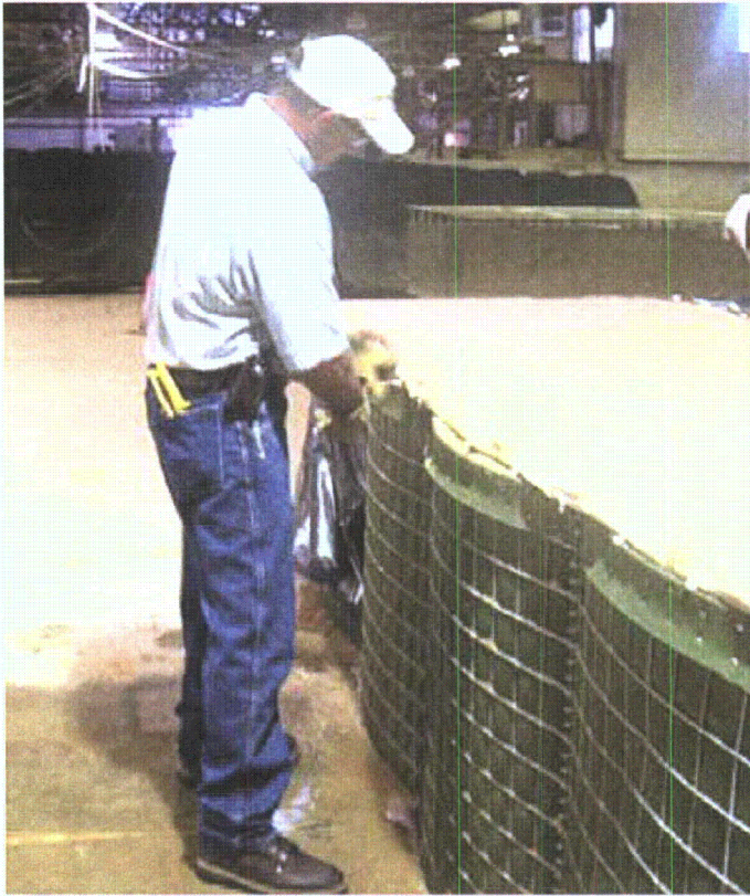
Figure 2-89. Cutting cable ties and removing top cover
