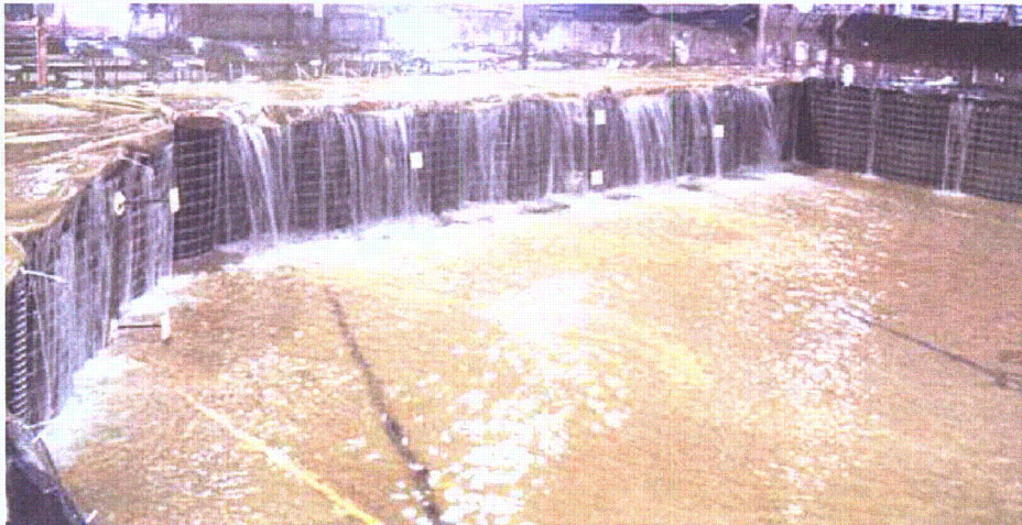
Figure 2-84. Overtopped levee structure, view from left wall
