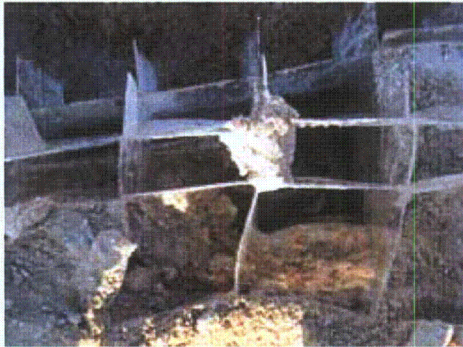
Figure 3-122. Fill material washed out of units (view down from top)
