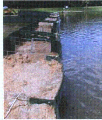
Figure 3-87. 11 June 2004, 4.0 ft of water against structure
