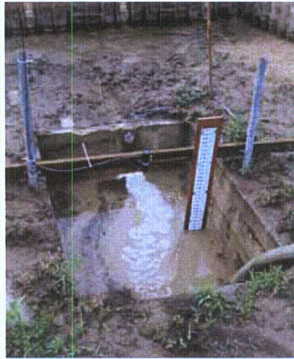
Figure 3-121. Seepage collection in sump tank
