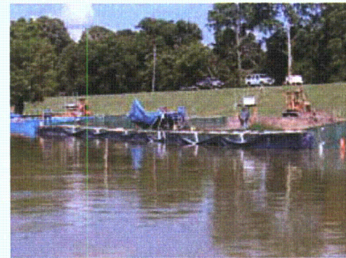
Figure 3-85. 9 June 2004, 3.1 ft of water against structure
