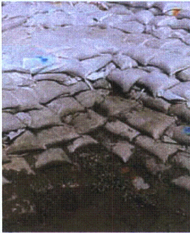
Figure 3-52. Seepage through structure
