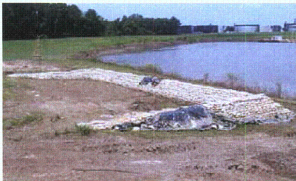
Figure 3-57. Structure after being submerged
