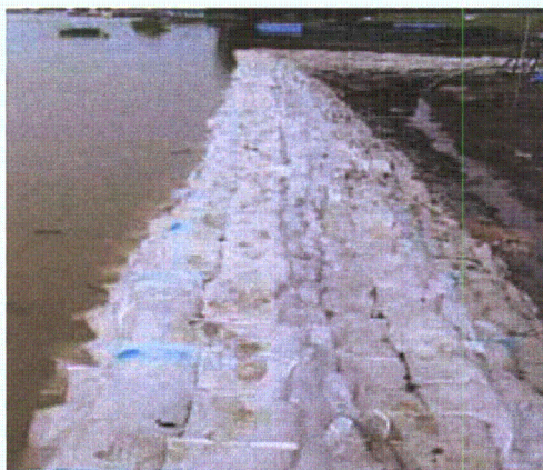
Figure 3-47. 6 June 2004, 3.3 ft of water against structure
