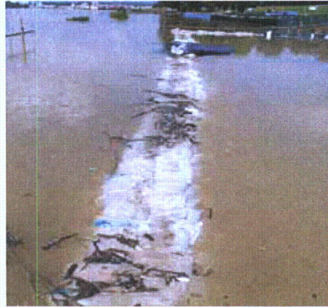
Figure 3-50. 7 June 2004, overtopped structure
