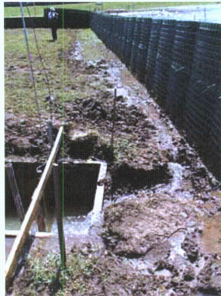
Figure 3-90. Seepage on protected side
