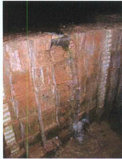
Figure 3-129. Overtopping of RDFW structure
