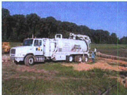
Figure 3-135. Rented vacuum truck
