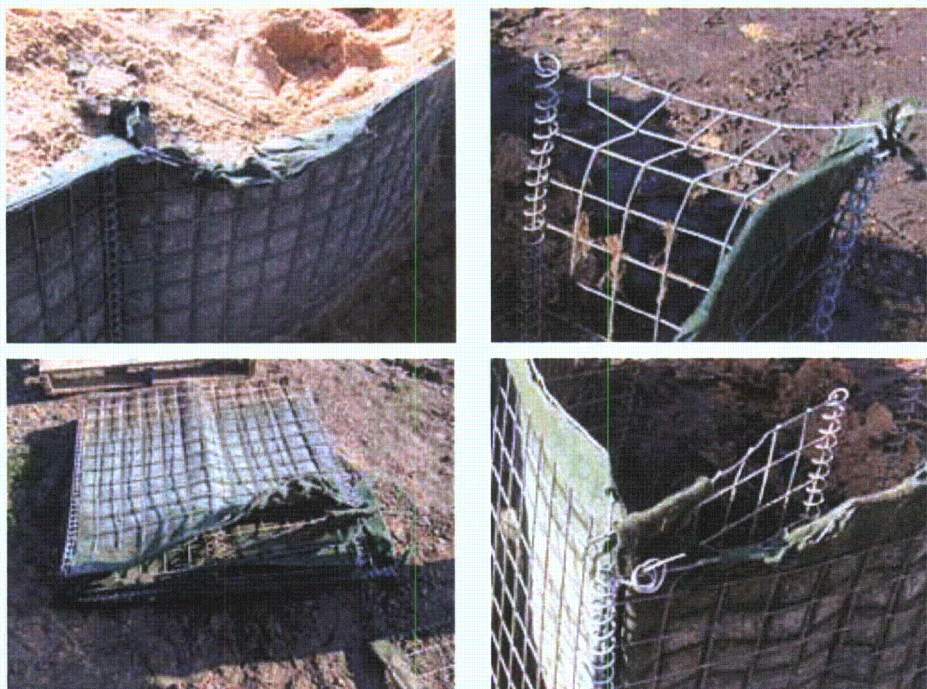
Figure 3-104. Units damaged during removal process
