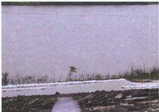
Figure 3-38. Rain water collected inside structure
