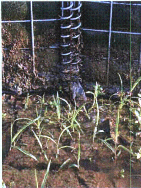
Figure 3-89. Seepage through joints
