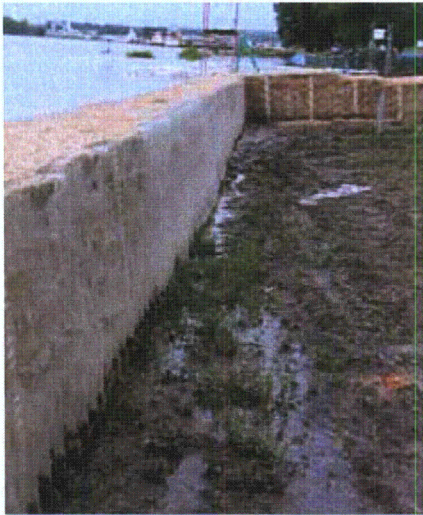
Figure 3-120. Seepage behind RDFW structure
