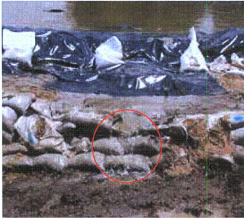
Figure 3-49. 7 June 2004, seepage through structure
