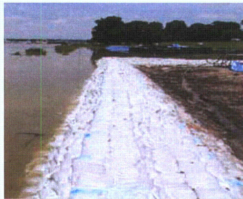
Figure 3-46. 5 June 2004, 2.3 ft of water against structure
