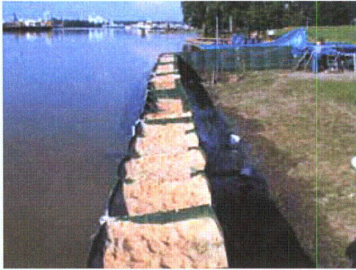
Figure 3-86. 10 June 2004, 3.5 ft of water against structure
