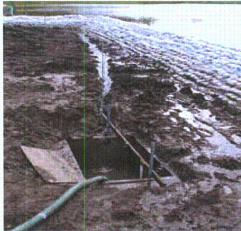
Figure 3-53. Seepage on protected side
