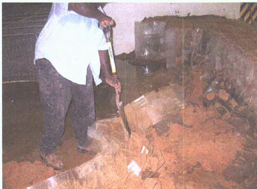
Figure 2-164. Shoveling out sand/cement mixture from toe grid units and pulling out grid
