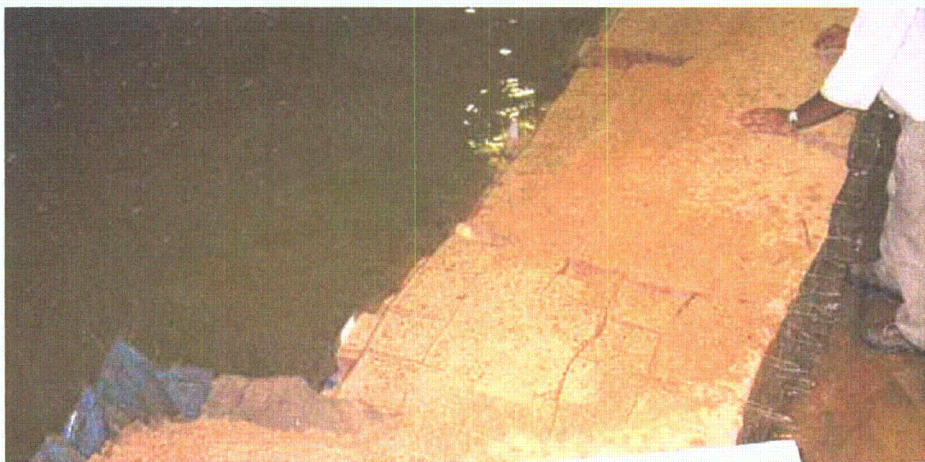
Figure 2-143. Surface erosion from wave action
