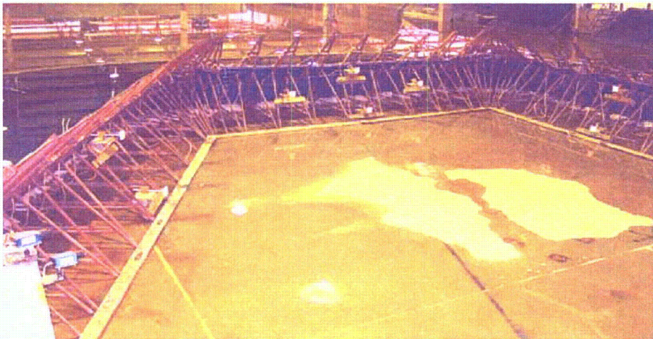
Figure 2-216. Under-apron seepage at 1-ft hydrostatic test
