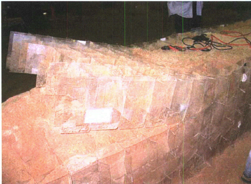
Figure 2-173. Loosened grid unit
