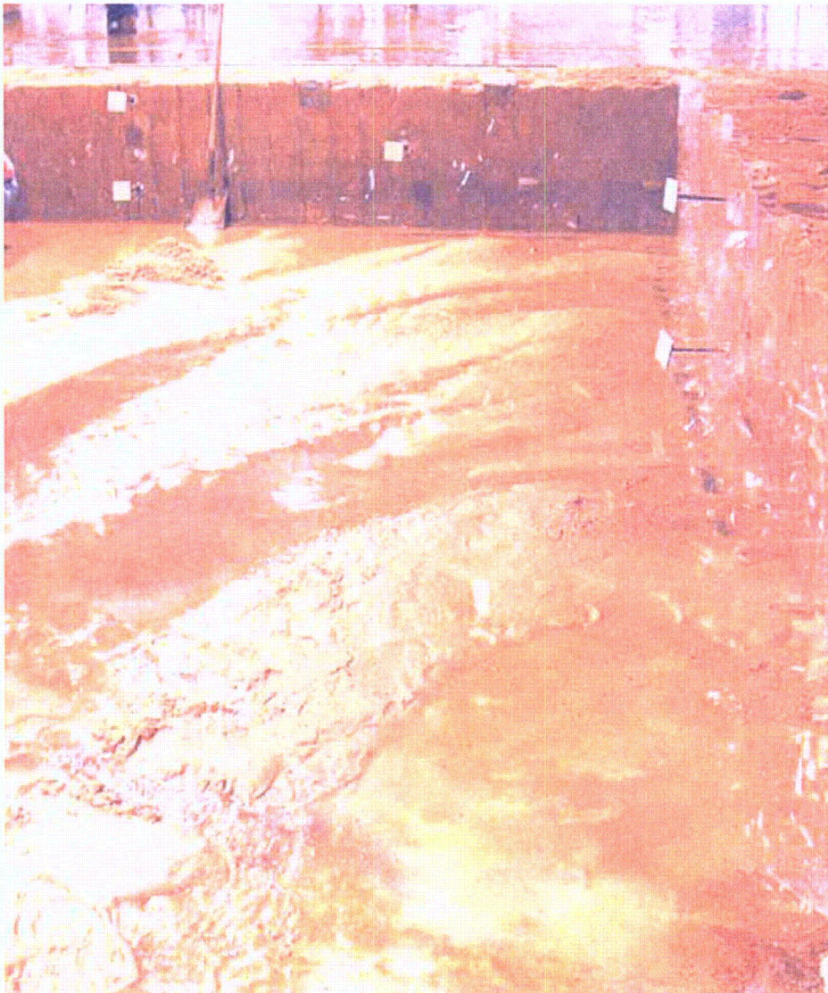
Figure 2-159. Eroded sand deposited on floor (view toward center and right walls)
