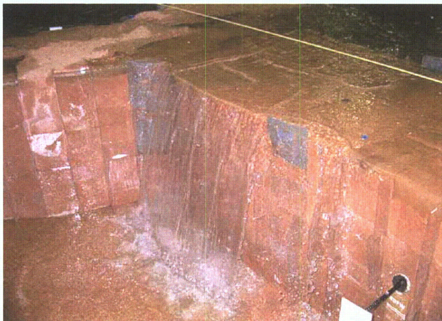
Figure 2-147. Sporadic wave overtopping at intersection of left and center walls
