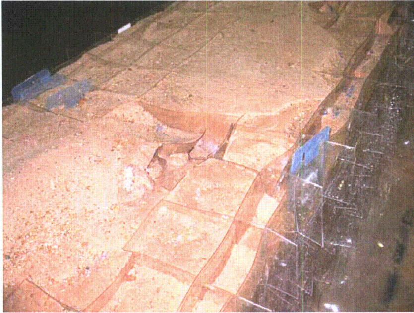
Figure 2-150. Close-up of surface erosion on left wall
