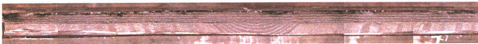
(b) Appearance of fracture surface of channel head body after removal of sample
