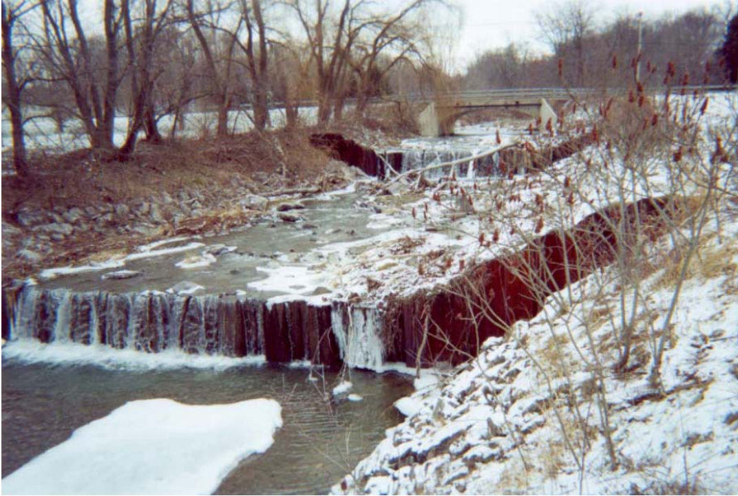
Figure 6.6 A functioning drop structure. The steel ledges prevent water from flowing too quickly down this stream.
