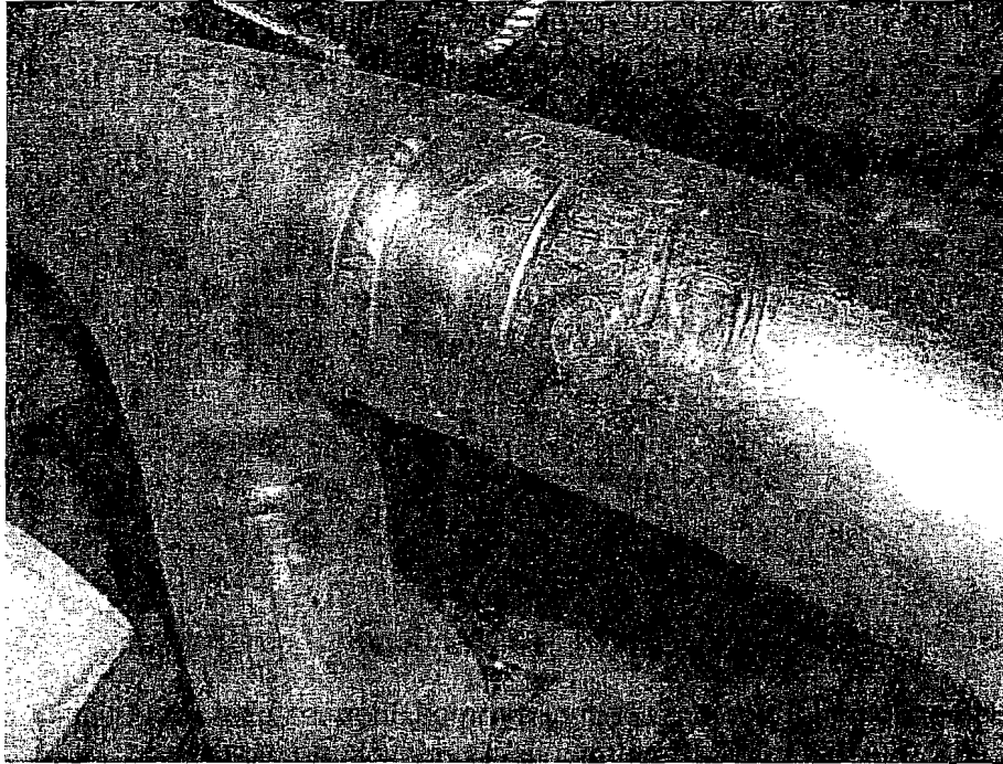
Figure 1: Wear indications identified on CVCS Letdown Piping
