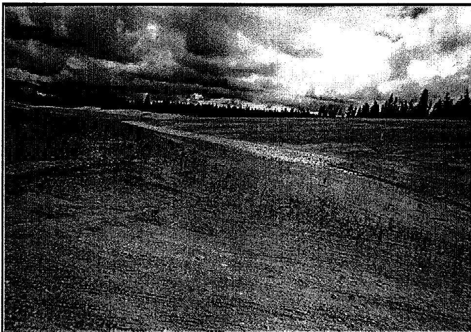
Location 21, looking N showing ending section of diversion dike and margin toe rock protection. Some erosion is evident parallel to toe.
