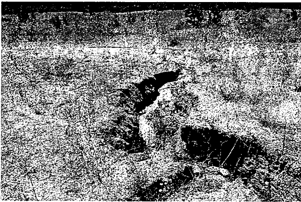
Photograph is of gully formed at the south end of the impoundment surface, between the swale and east margin. Runoff from this general area toward the south has cause this gully.
