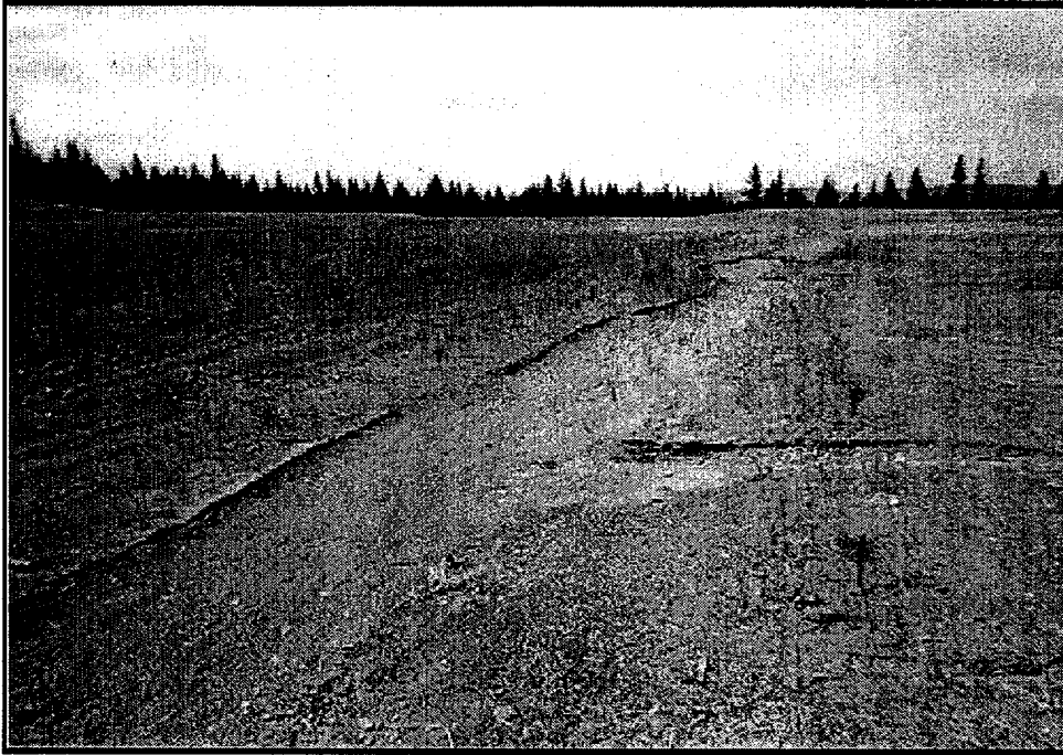
Location 23, looking S showing erosion from upstream of swale. Main channel is from N., side channel is from E (impoundment surface), depths to 4 inches.
