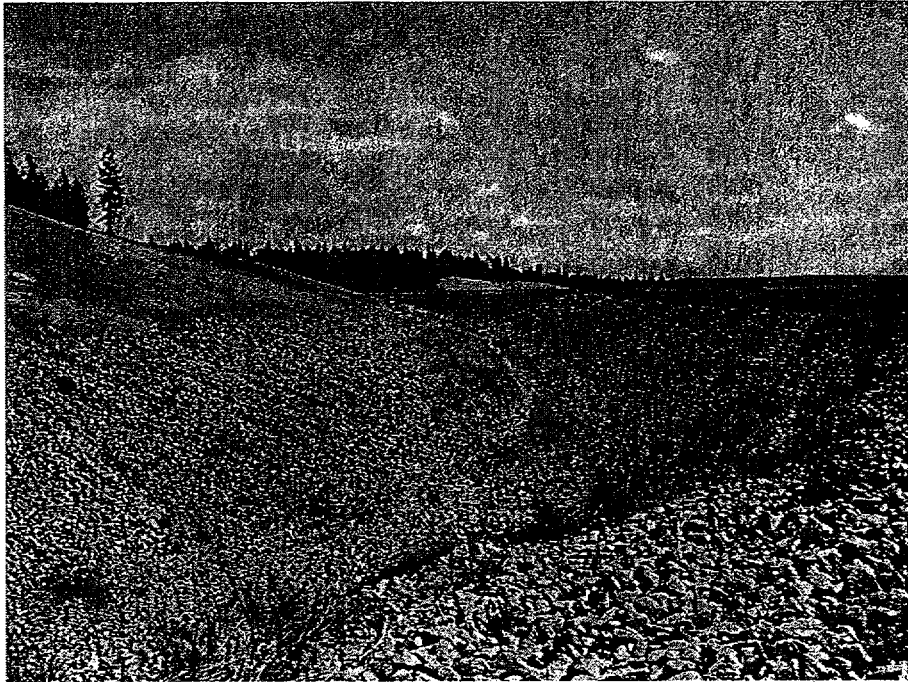
Picture 34: Looking downstream towards Confluence F. The water in the channel is from a spring intersected during construction.
