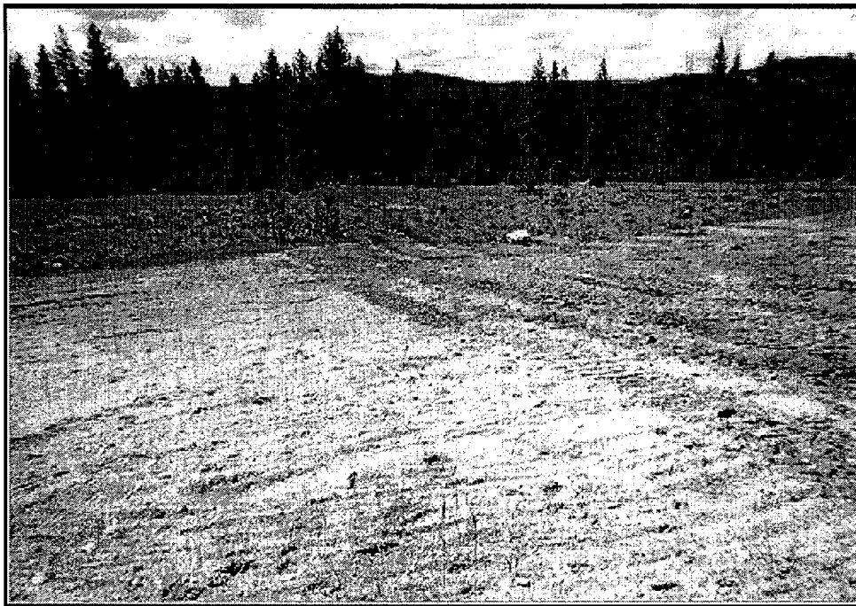
Location 21, looking S showing rework from early spring erosion and transition to natural vegetation.
