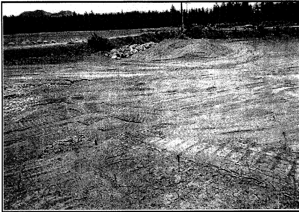
Location 12, looking S from power pole near truck shop vehicle access road culvert (mill site).
