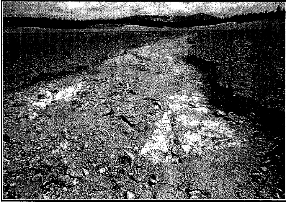
Location 22, looking N from swale outfall (up slope) showing erosion to about 1 foot and local underlying rock and bedrock outcrops.
