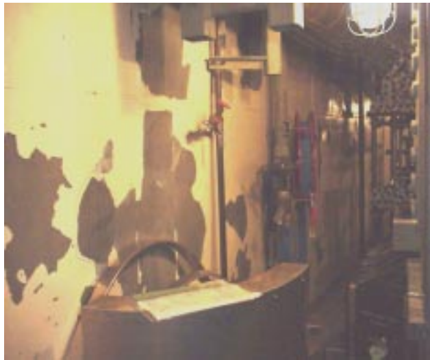
Examples of Failures of a “Qualified” Coatings System Phenoline Topcoat with CZ11 Primer on Steel Liner
